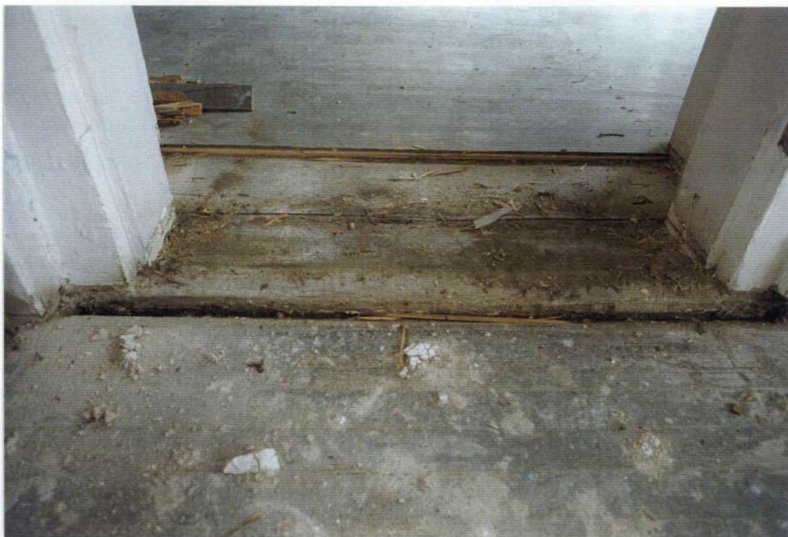
114. Space 102 to 103 Door frame mortise and tenon pegged door threshold.
