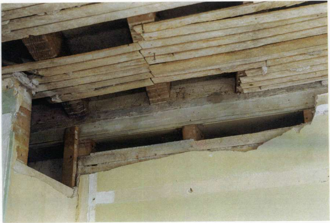
164. Detail: west wall, north side of fireplace chimney breast showing uncut original beaded corner beam. Note where original wood lath and plaster ceiling abutted side of beam.
