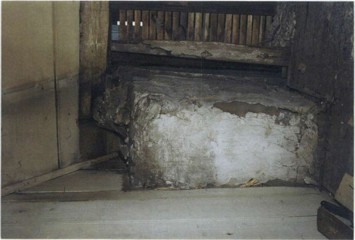
148e. Space 204C. Southeast corner of phase one stone wall at garret level. Note phase two roof sill plate.
