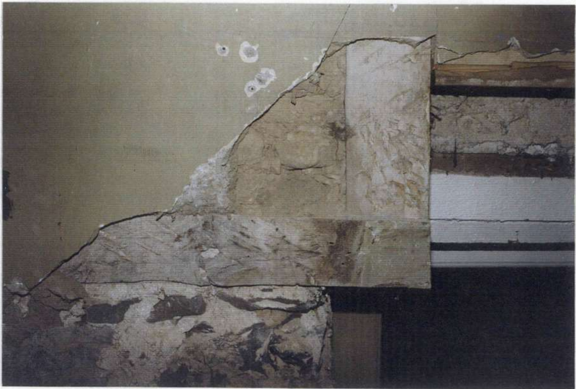
135b. Space 104. West wall after removals. Sill plate for wood framed phase three structure with hand-hewn posts and brick infill. Left side of door to phase two cellar.
