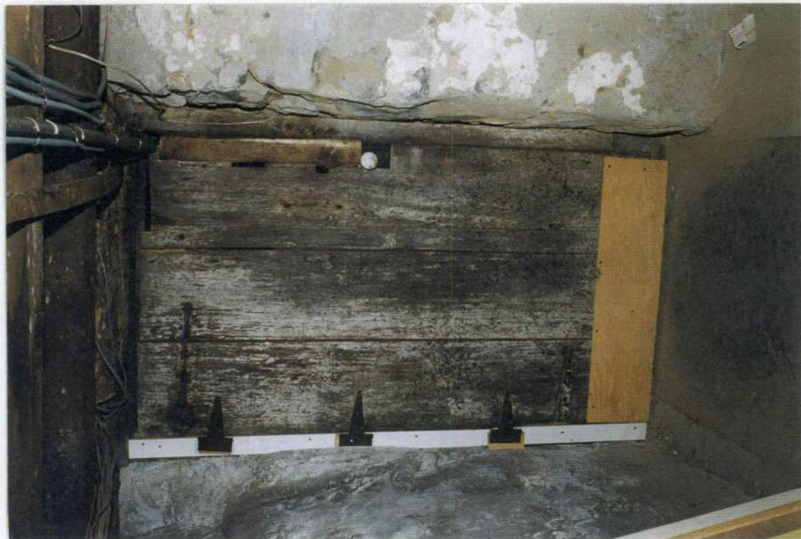
155. Cellar door between space 001 and 003 as seen from space 003. Door shows shadows of Dutch pancake strap hinges. Stone wall to right of door reinforced with stone and butterssing original east wall of phase one exterior side.
