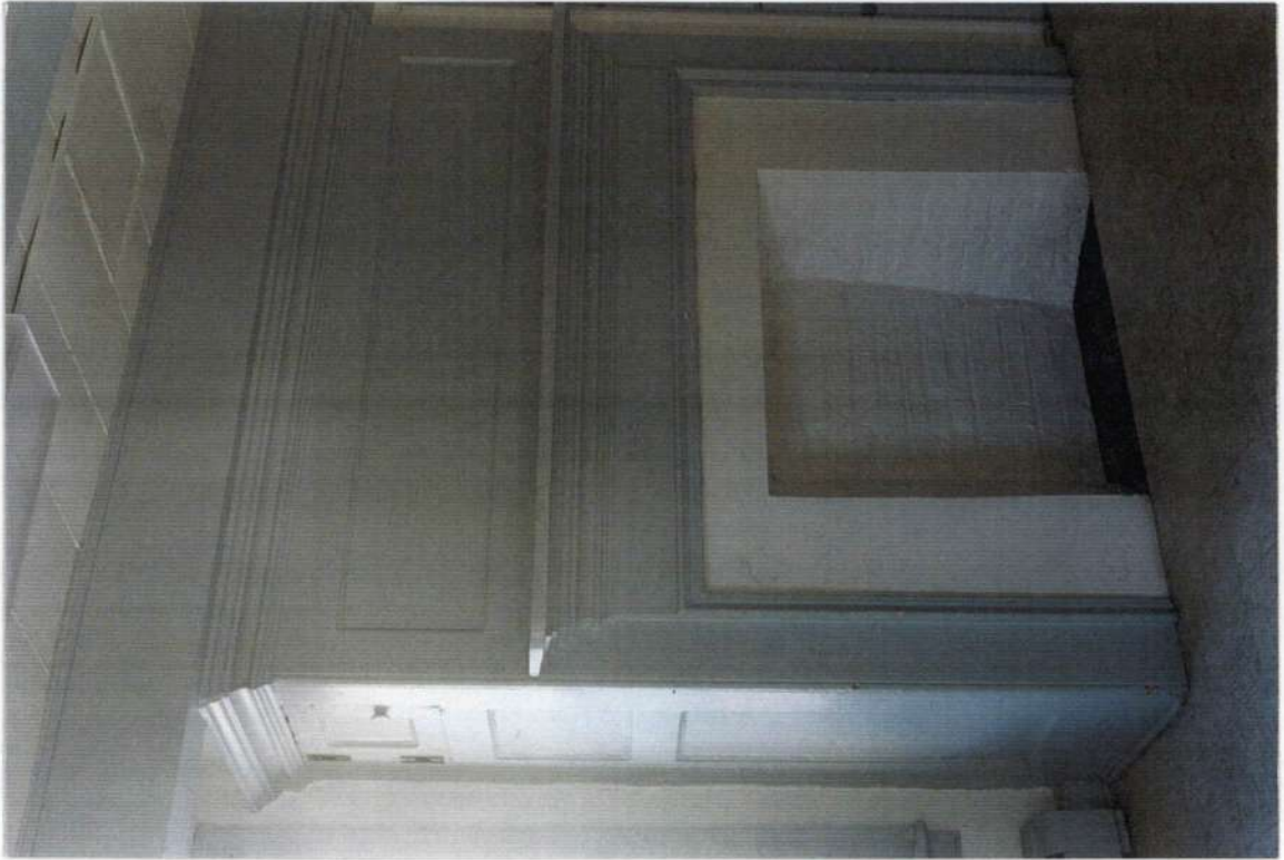
46. Space 101 north wall. Detail of English style paneled fireplace with heavy cornice moulding.
