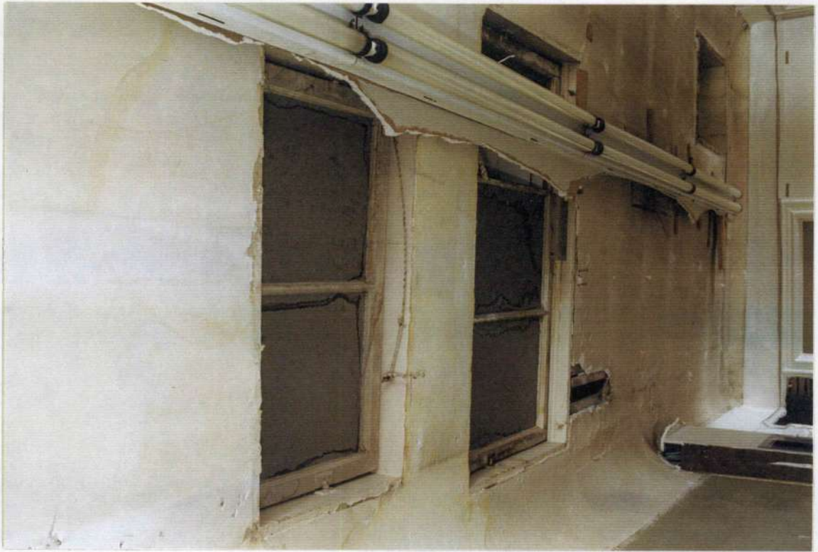
246. Space 211 laylights in ceiling opening to roof covered over by recent dropped ceiling.
