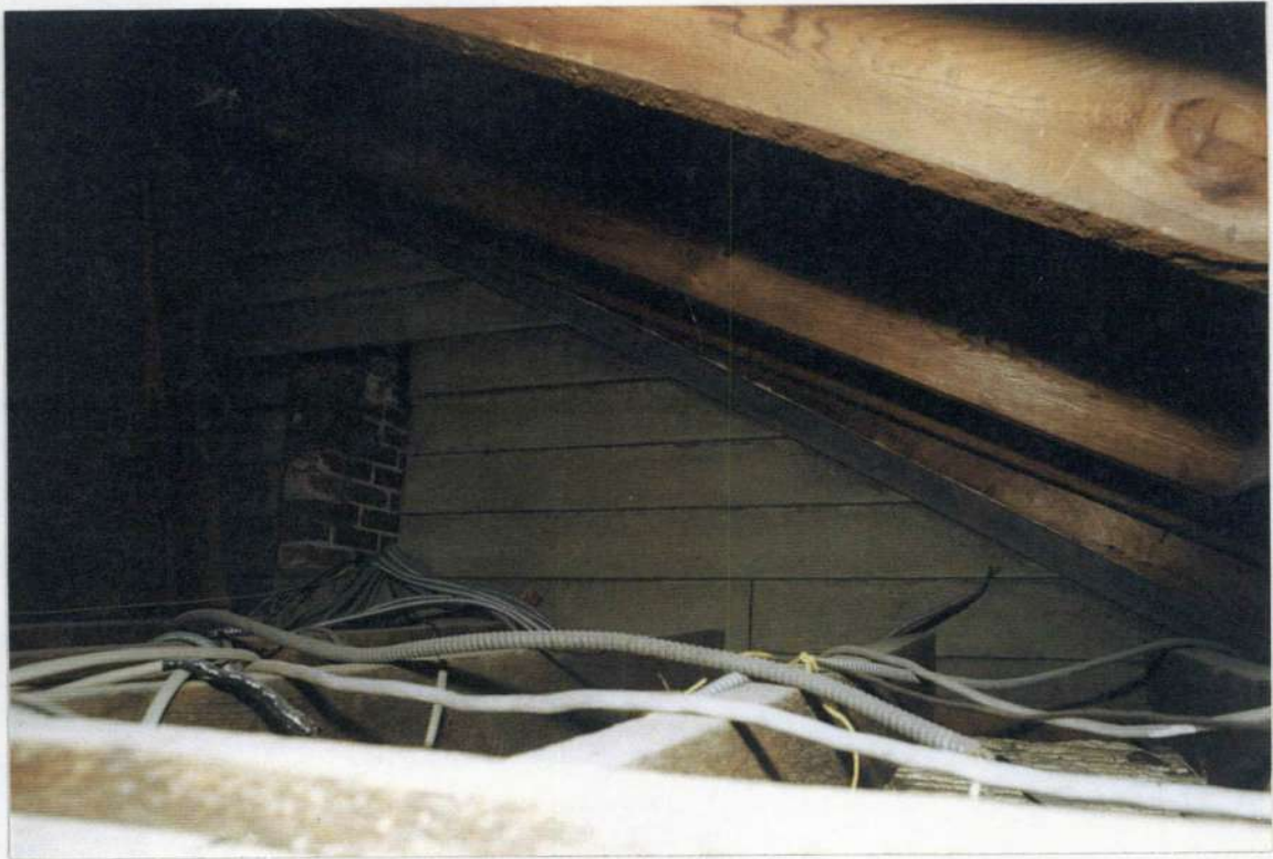
152e. East wood framed exterior clapboard gable ended roof of phase three as seen from phase five attic.
