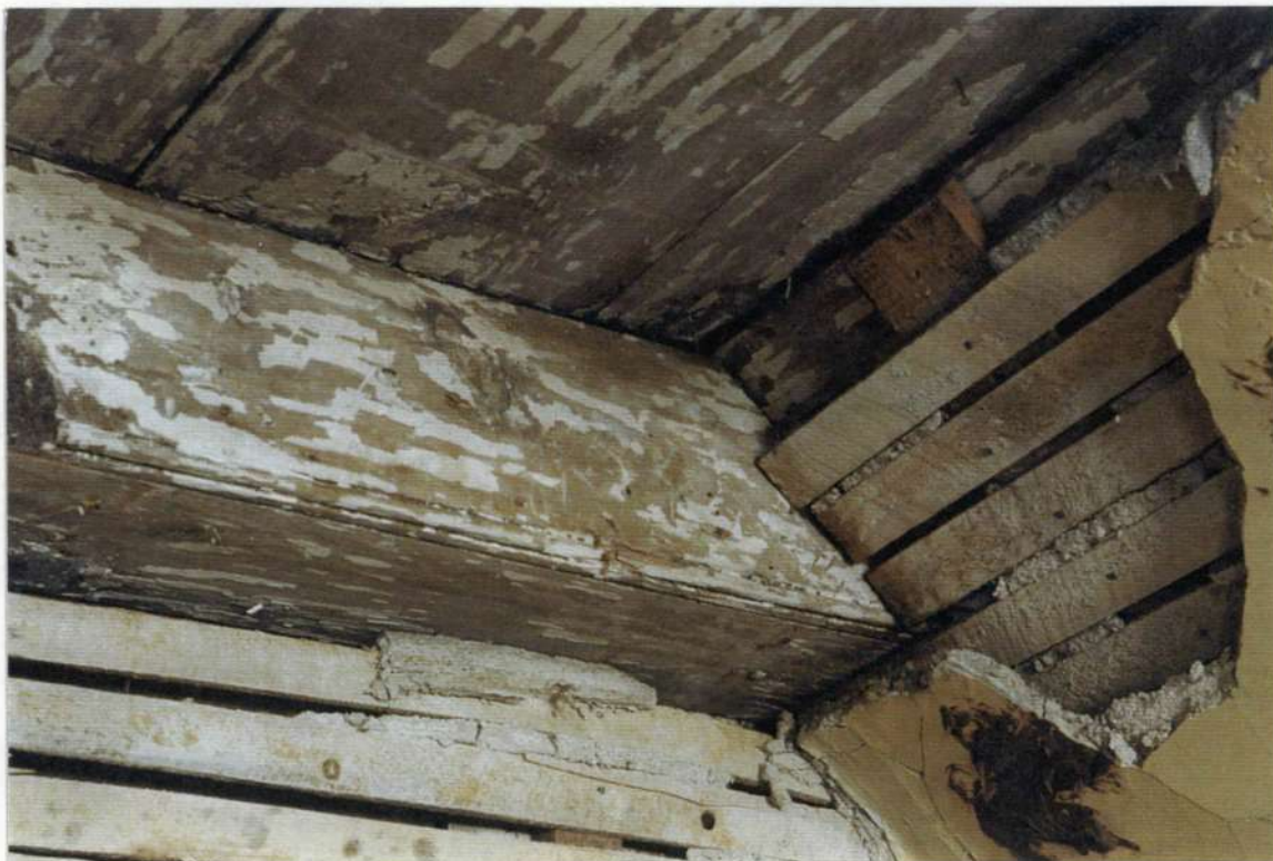
81. Detail: Space 201 southwest ceiling corner showing original boxed trim collar beam and wood plank ceiling with wood lath and plaster ceiling and wall added over earlier wood plank.
