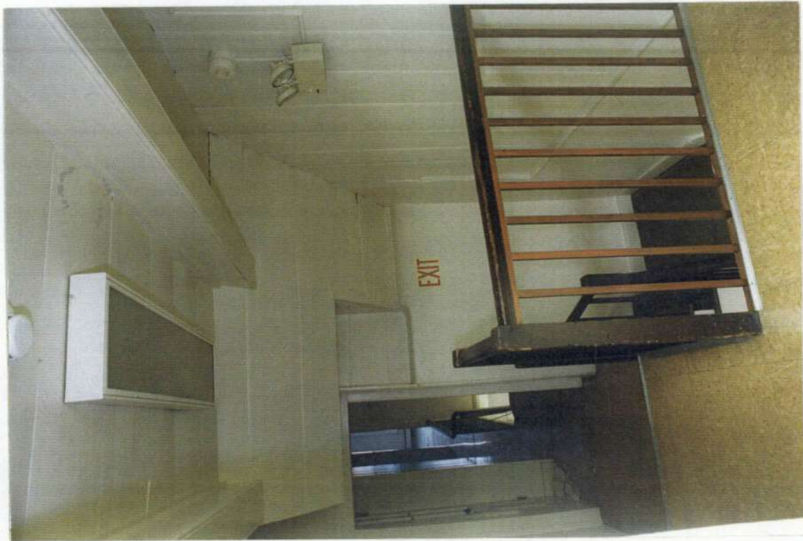
63. Space 202. Stair hall looking east. Note vertical board wall and ceiling. Ceiling collar beams with boxed trim detail.
