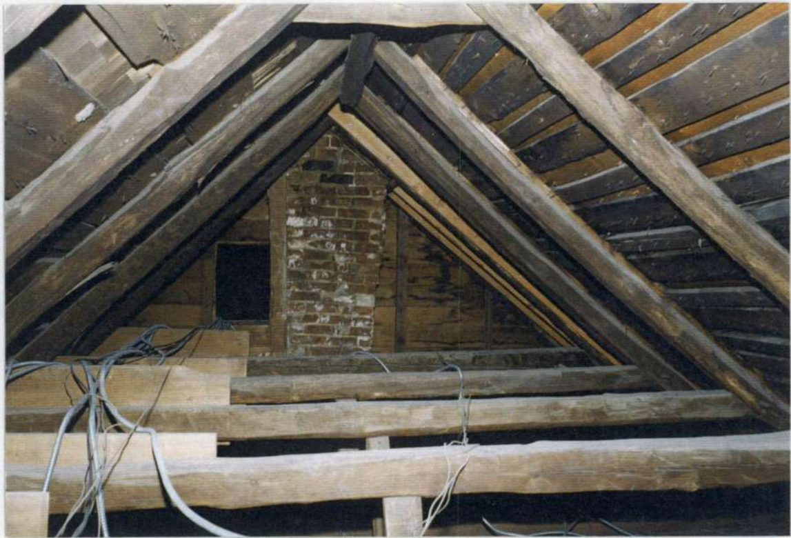
149. Attic over space 205 looking east at brick chimney. Note ends of sistered collar ties (left).
