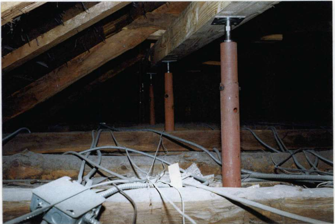
222. Attic over space 208 looking west. Note emergency shoring for failing roof along east stone wall.
