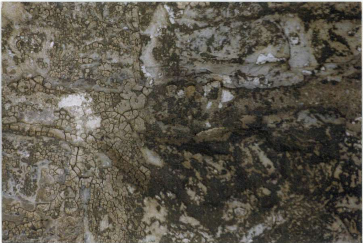
37. John Street detail at right of entry door where ca. 1850s gothic revival decorative hood was removed leaving impression of earlier paint below.
