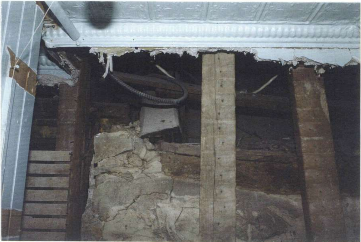
148d. Space 205A. Southeast exterior corner of phase one roof framing. Note sill plate and last rafter. Phase two east roof sill plate seen to left.
