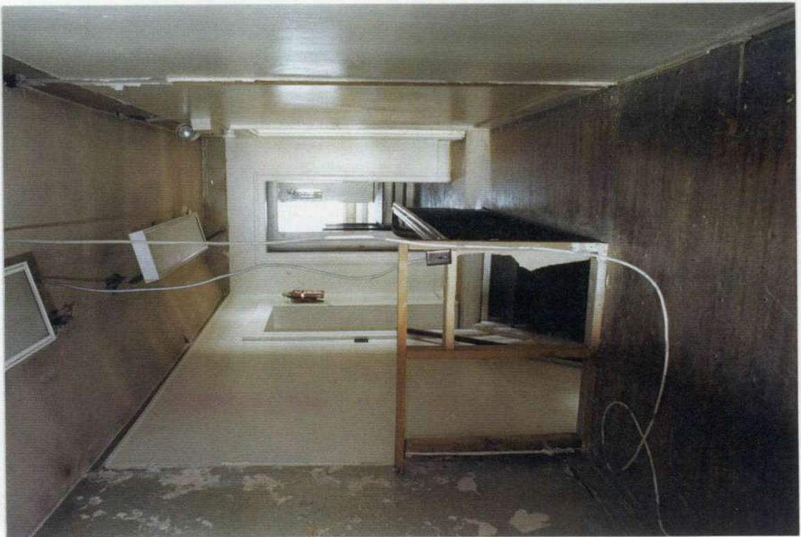
192. Space 210 looking west after removals. Note plaster on stone wall on left.
