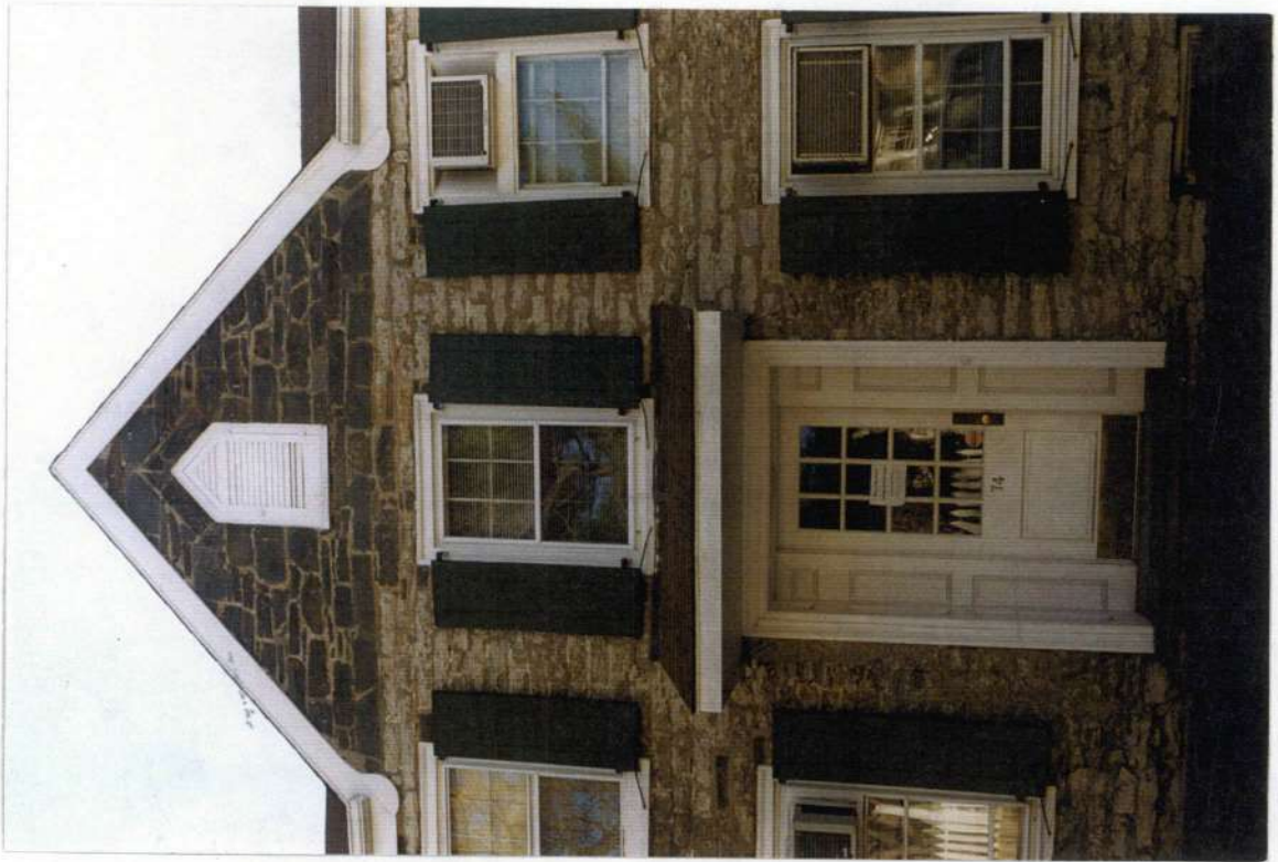
28. John Street ca. 1850s gothic revival stone gable and louver opening addition. 20 th century entry door with ca. 1970s hood roof.
