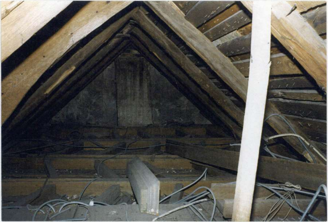
125. Attic framing over space 204. Note collar ties at floor above wood lath and plaster ceiling. Note abandoned mantel; note plastered chimney and south end wall.
