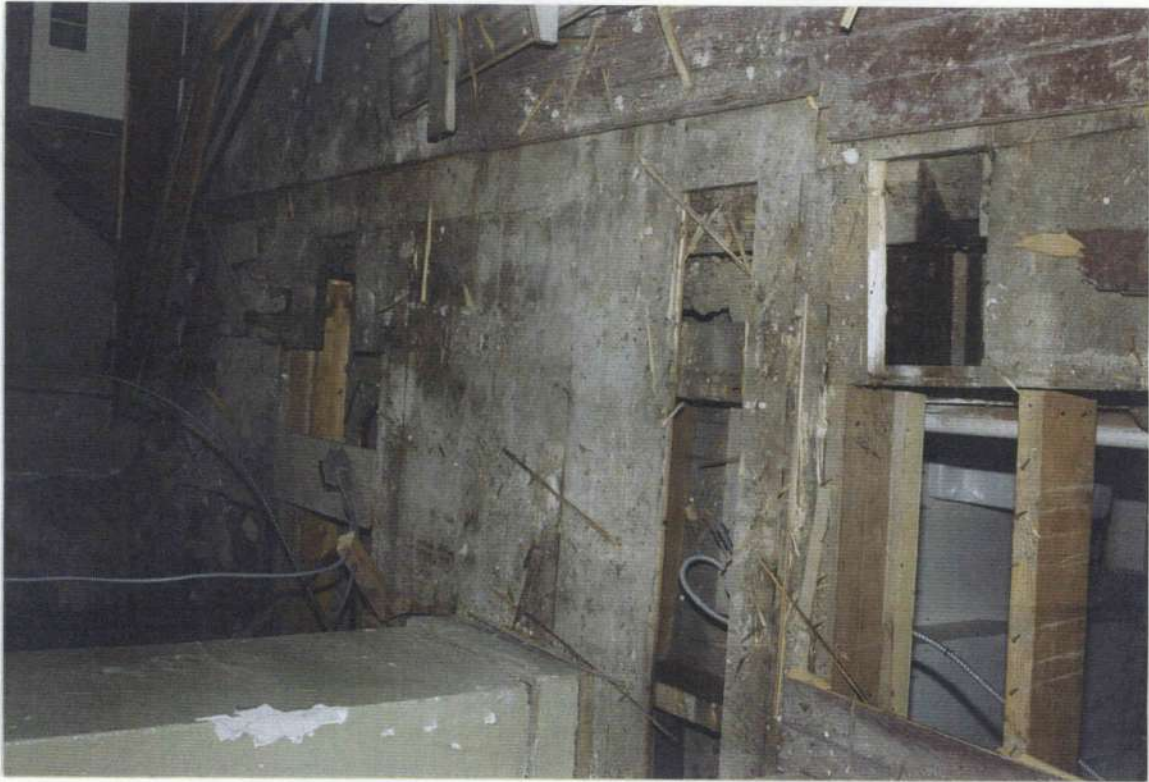
148k. Space 205. East wall looking south. Area where stone wall and fireplace of phase three removed in phase five.
