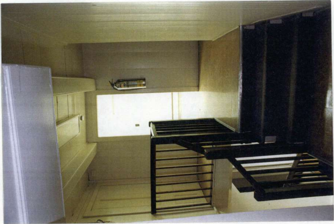
62. Space 202. Stair hall looking west. Stair steps down from phase one to phase four second floors.
