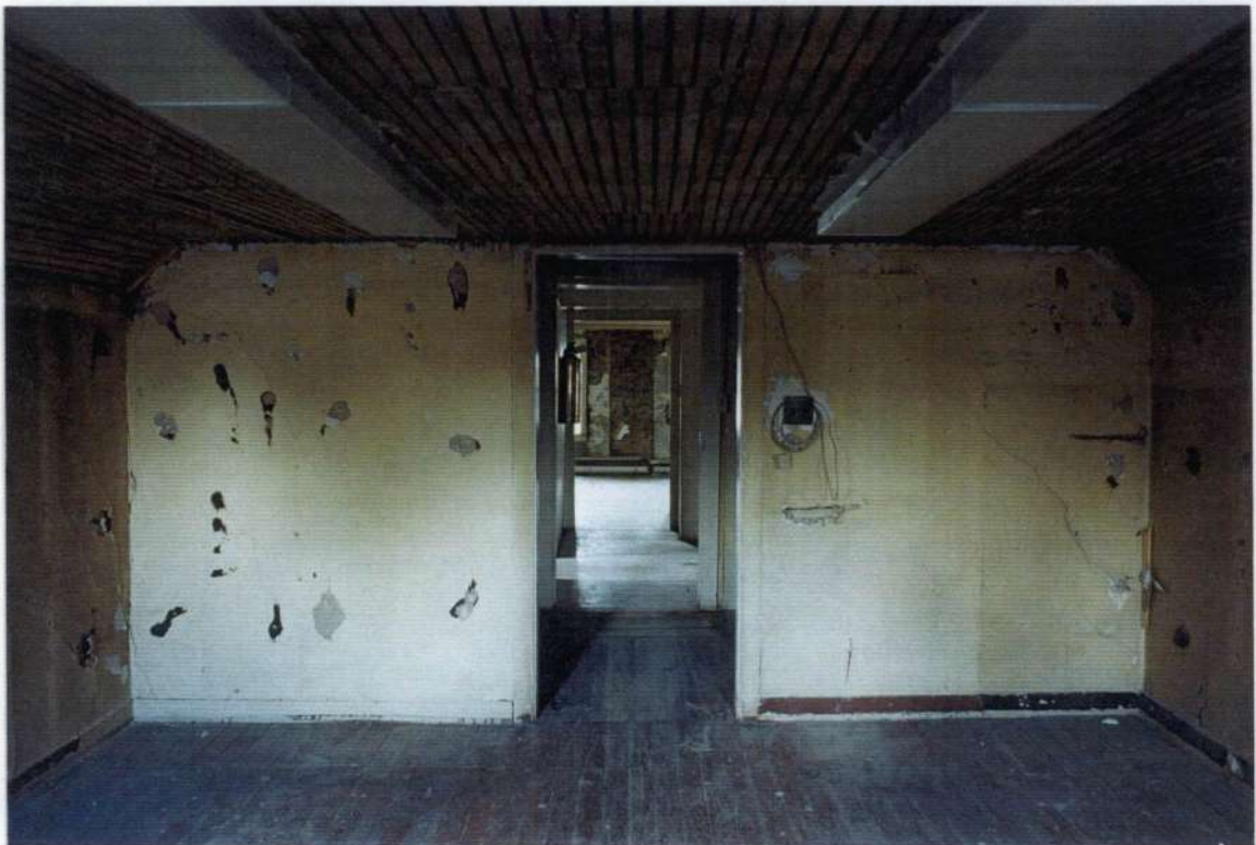
119. Space 204. North wall after removals. Note wood lath and plaster ceiling on sloped and flat ceiling.
