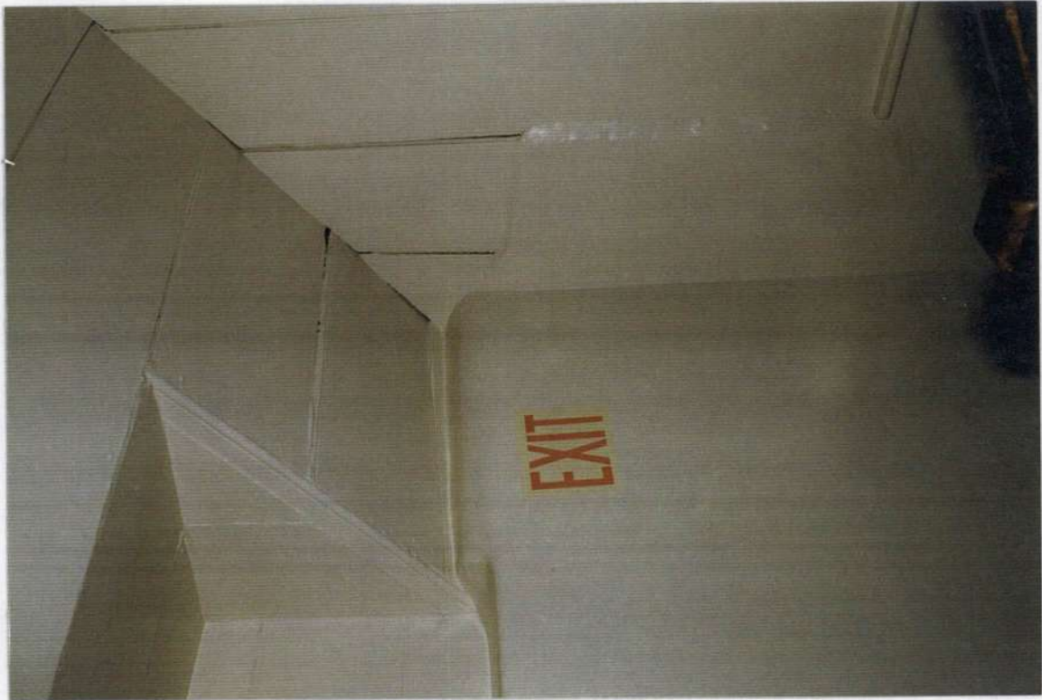
64. Space 202. Second floor phase one stone wall and wood ceiling juncture. Note knee wall common to phase two removed except at corner.
