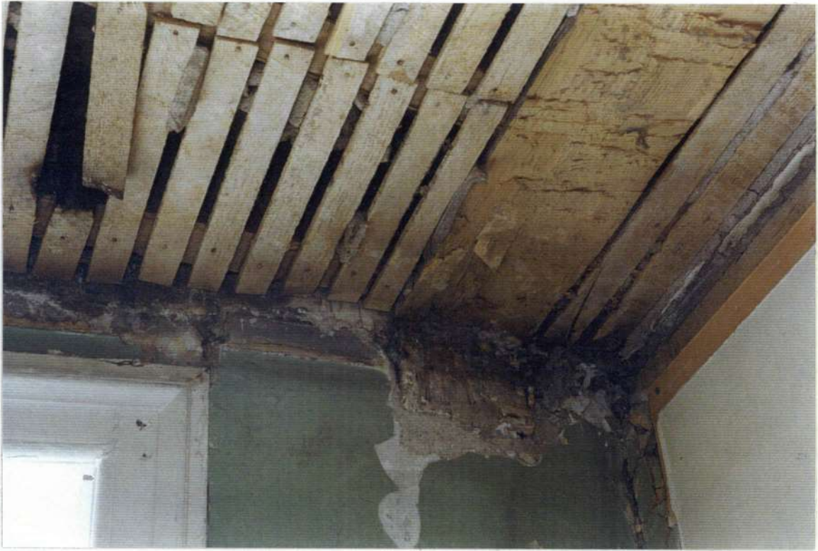
170. Detail: northeast end of north wall space 105 showing cut beam bottom, and line of early wood lath and plaster ceiling.
