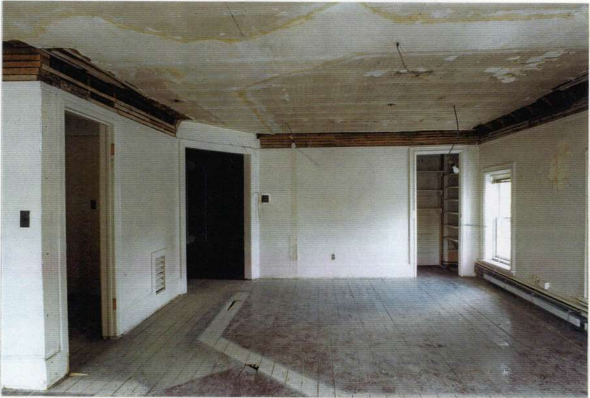
248. Spaces 213, 215, 216 looking north after removals. Note cove moulding at ceiling and wall.
