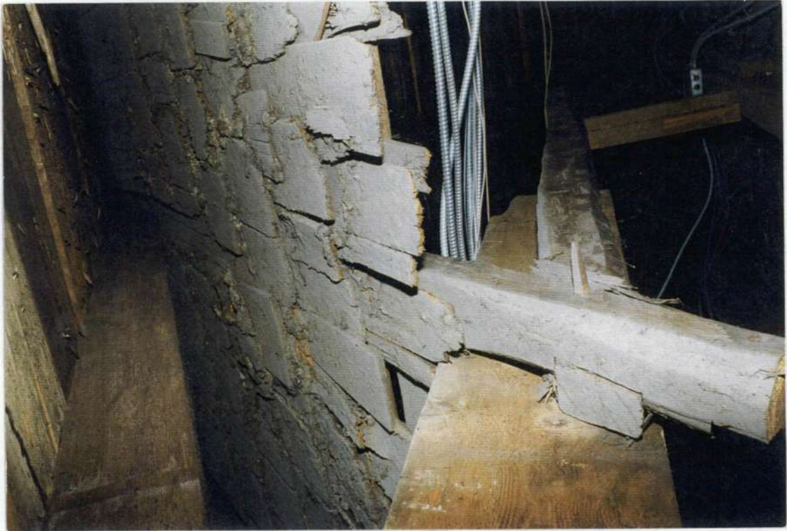
151. Abandoned 30" long hand planed shingle roof below phase five roof built over phase three roof. Note cut rafter end and sistered collar tie extension; phase five reframed roof is seen above.
