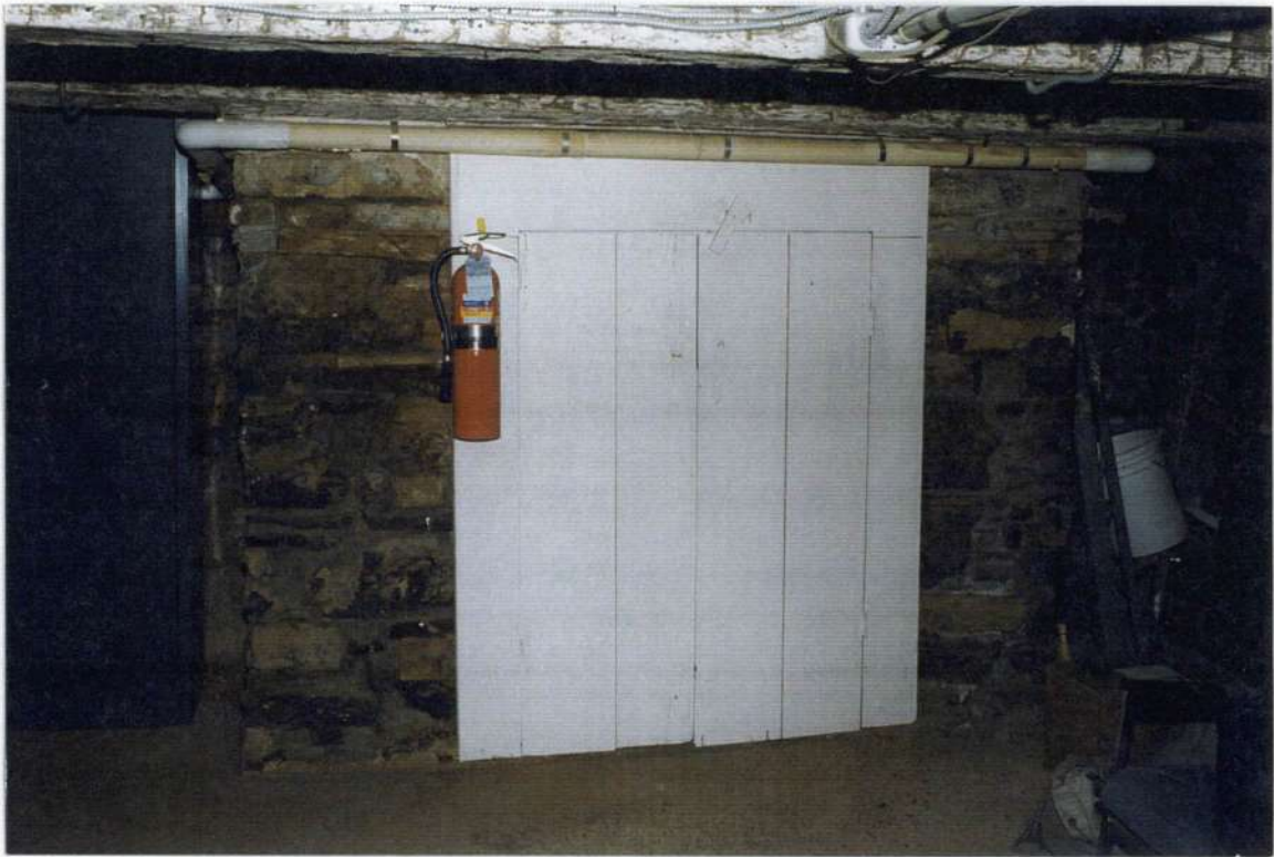
102. Space 002 south wall. Fireplace stone foundation and early plank doors over foundation opening.
