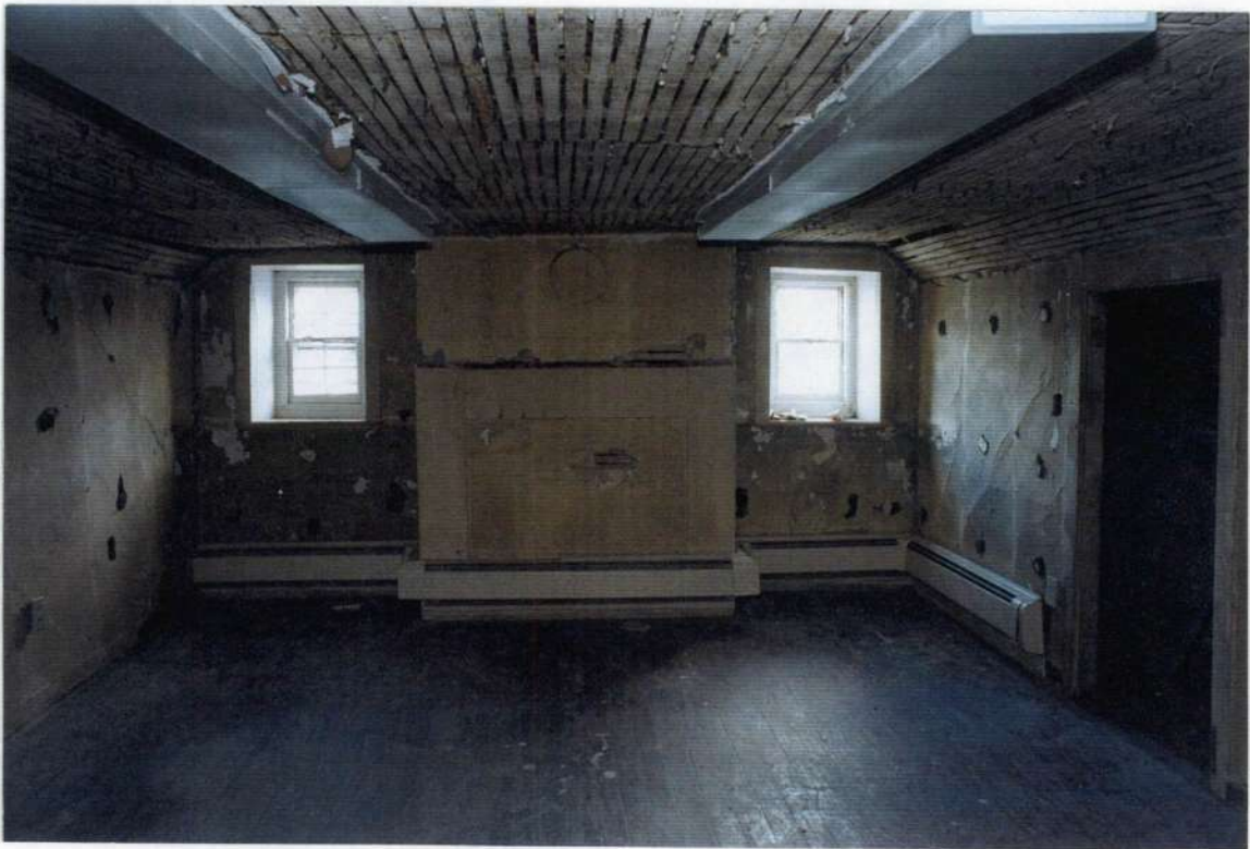
123. Space 204. South wall after removals. Note remains of plaster and lath built out chimney breast and mantel surround. Masonry chimney inside is similar to masonry chimney removed at north end phase one.
