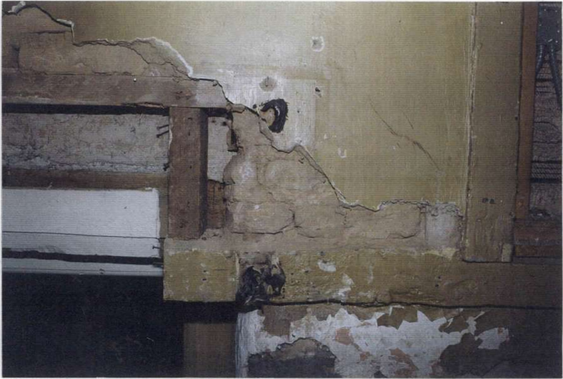
135a. Space 104. West wall after removals. Sill plate for wood framed phase three structure with hand-hewn posts and brick infill. Right side of door to phase two cellar.
