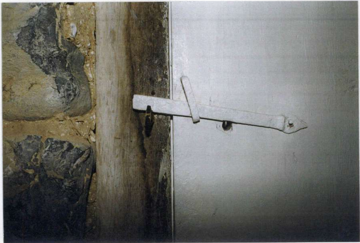
97. Detail: Wrought iron keeper latch.
