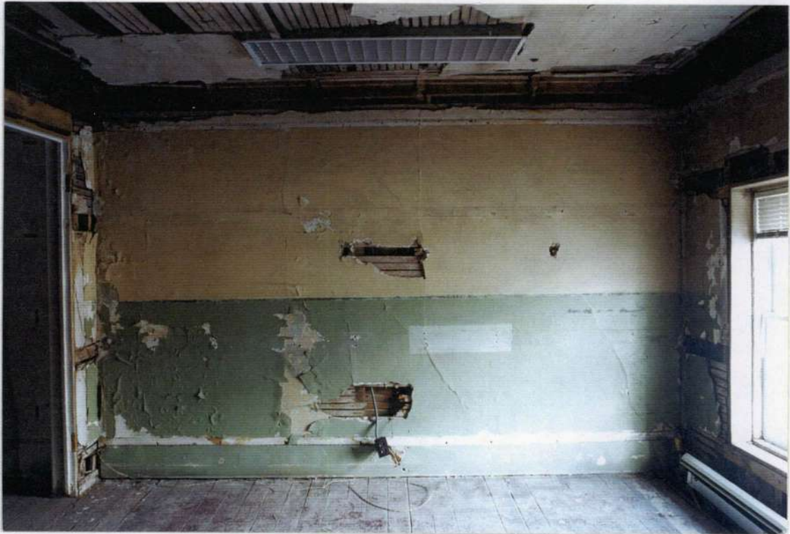
238. Space 212 north wall after removals. Wood lath and plaster furred wall over phase four exterior wall.
