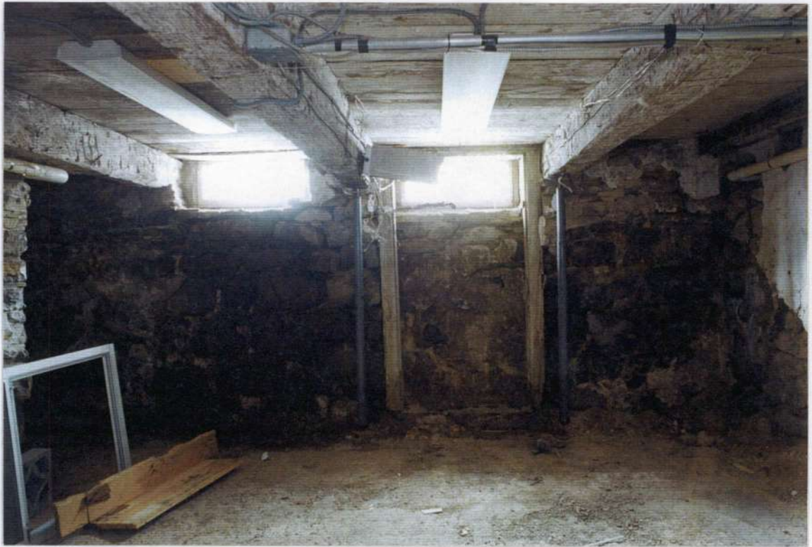
100. Space 002. West wall with cellar windows and abandoned mortise and tenon pegged door frame to Crown Street.
