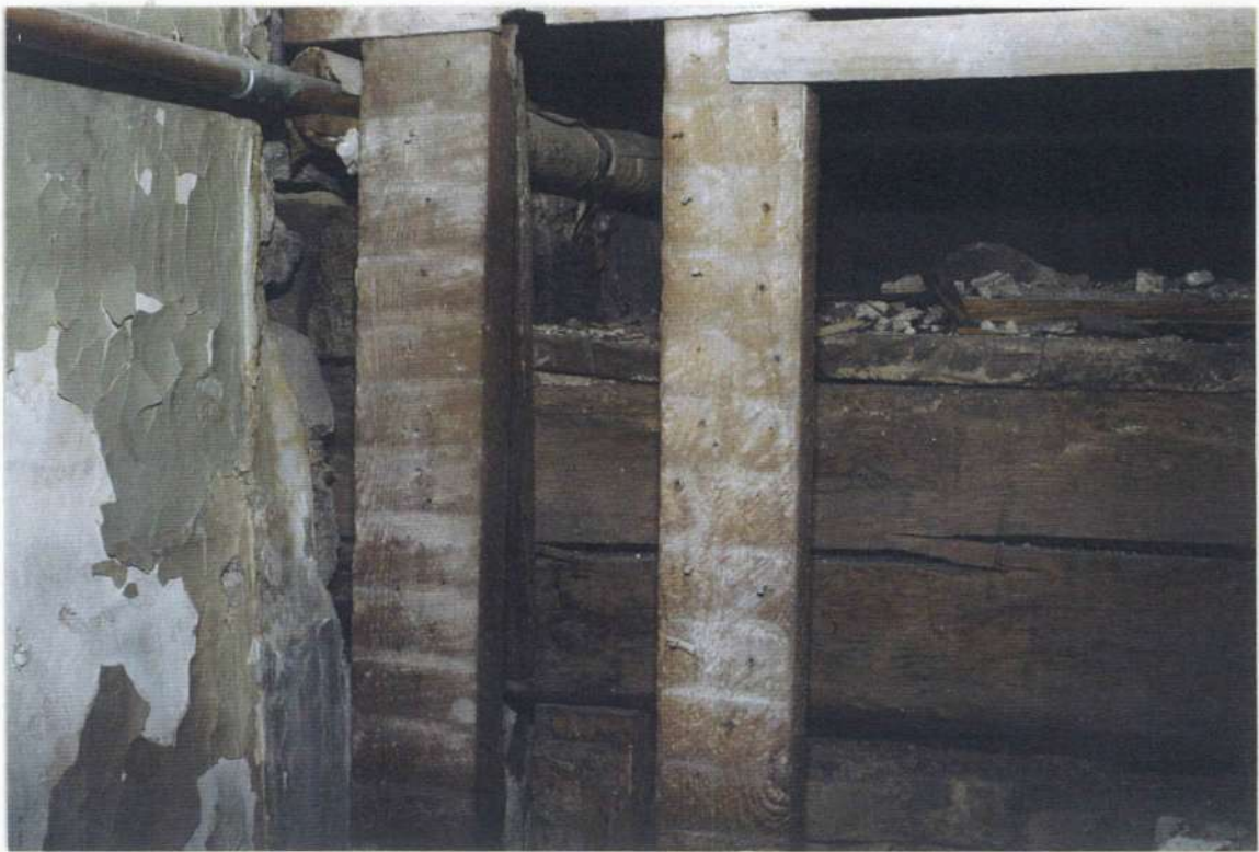
148b. Space 205. West wall after removals. (See note above) Note remains of hand-hewn beam in stone wall above top of phase two beam. Could be remains of phase three framing.
