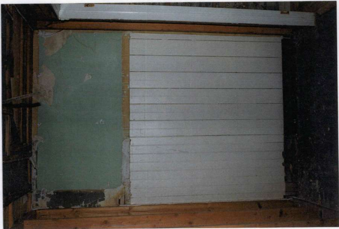
228. Space 111 north wall after removals. Note wood wainscot and plaster upper wall over early exterior stone wall of phase four.
