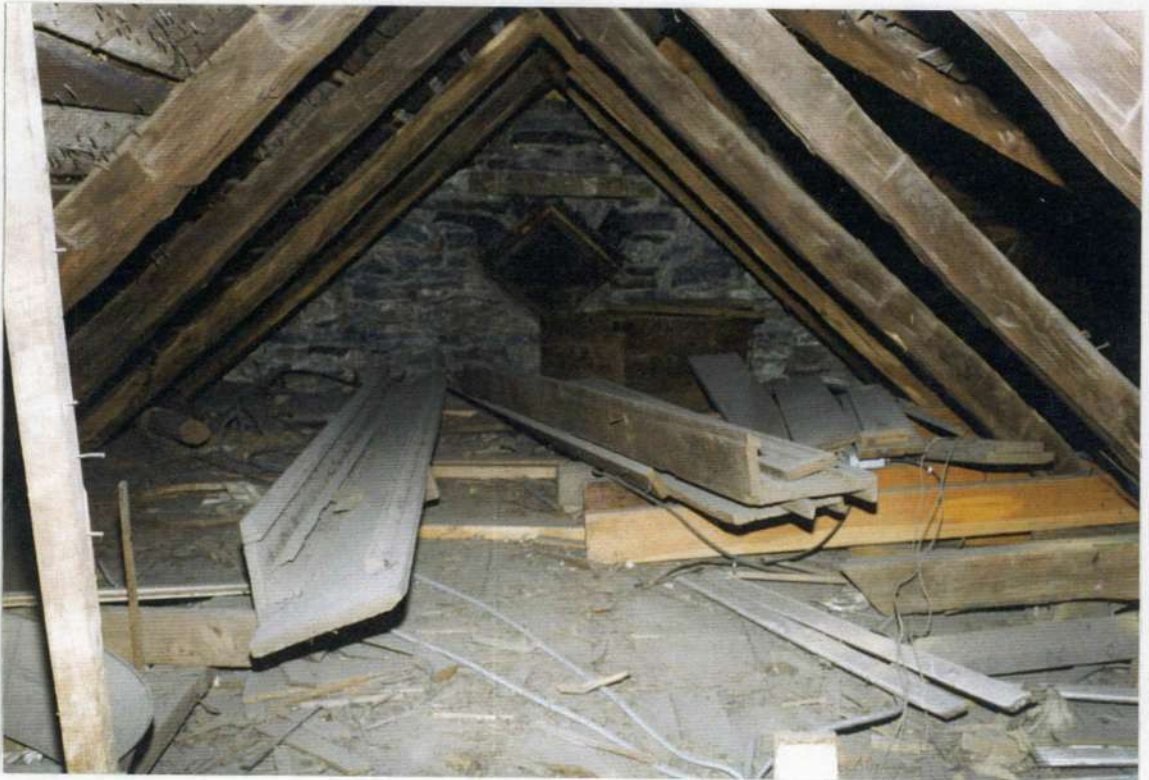
91. Attic of phase one over space 201 looking north. Note diamond detail in end wall where wood framed wall replaced. Brick chimney was removed in front of end wall with phase five renovation. Note remains of removed wood cornice board on attic floor.
