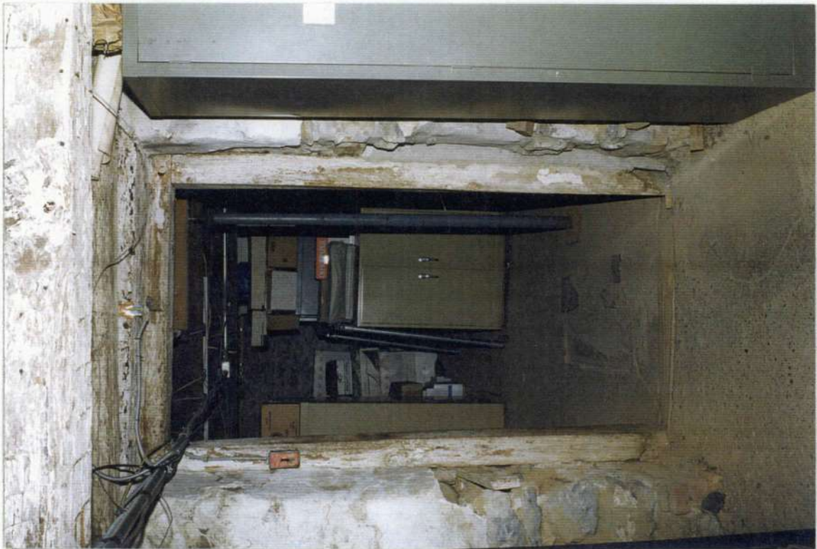
98. Detail: Heavy timber mortise and tenon pegged door frame between phase two and phase one as seen from space 002.
