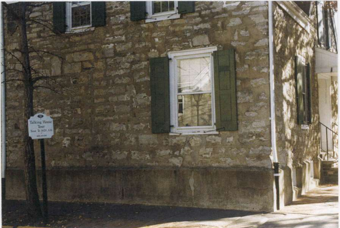
23. Applied concrete base to lower phase one wall at corner of Crown and John Streets.
