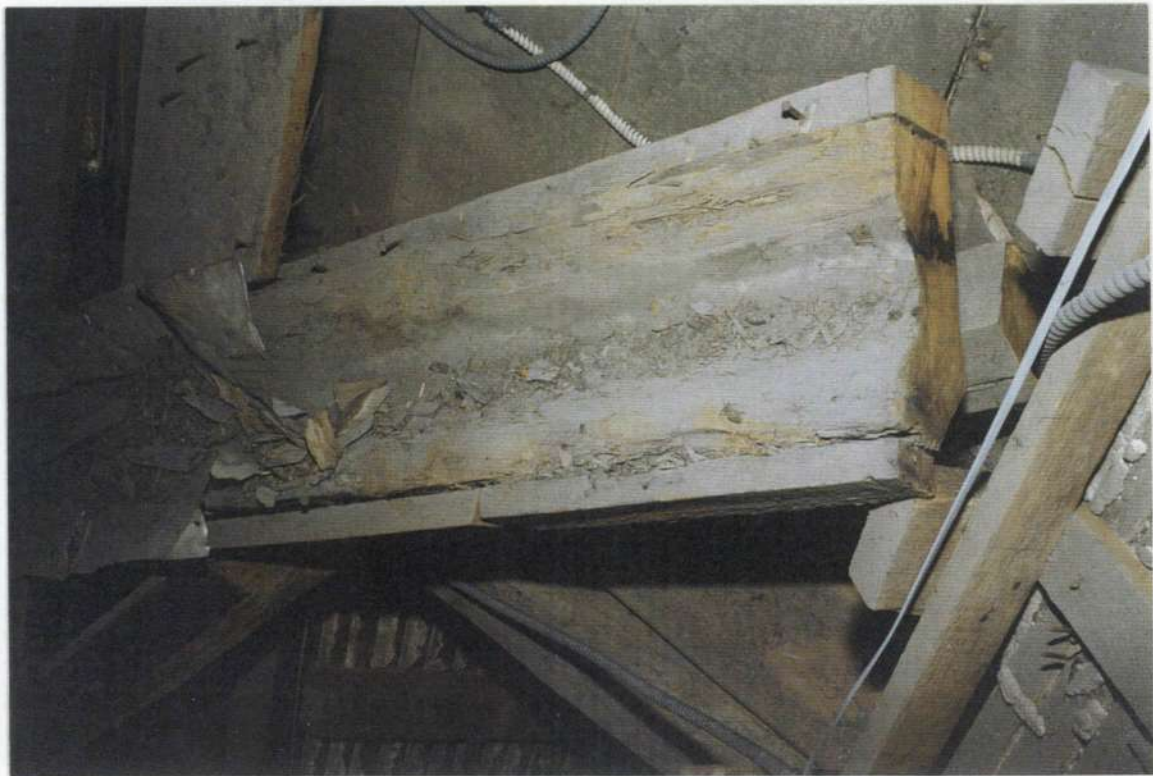
152d. Lower end of valley gutter above, sawn off at time of reframing of phase three roof, during phase four, and installation of plaster and wood lath ceiling.
