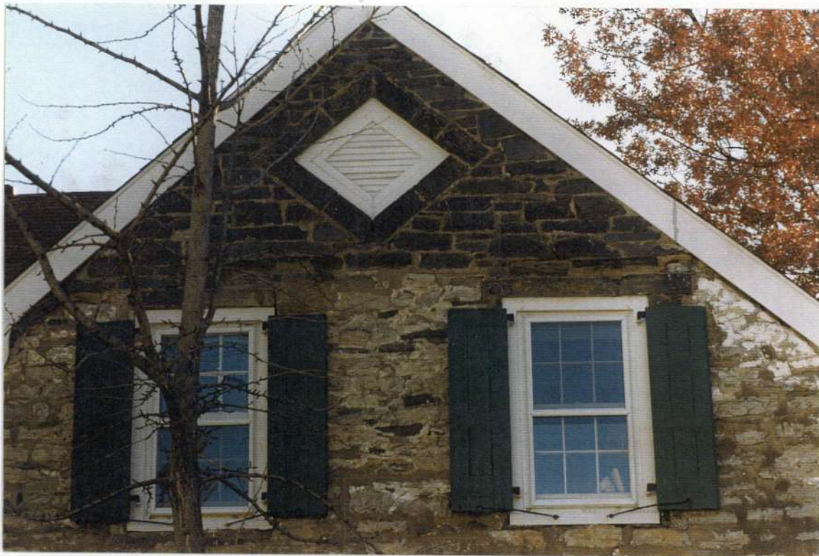
24. John Street gable end wall where darker stone replaced earlier wood gable end in ca. 1850s gothic revival period. Windows enlarged. Diamond detail added. Chimney removed. Dark stone was whitewashed to match earlier stonework.
