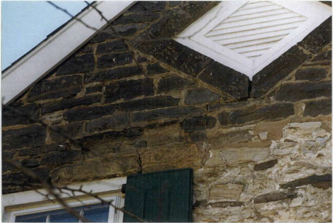
36. Upper John Street gable end of phase one where changes of stonework occurred that were whitewashed and eventually painted.
