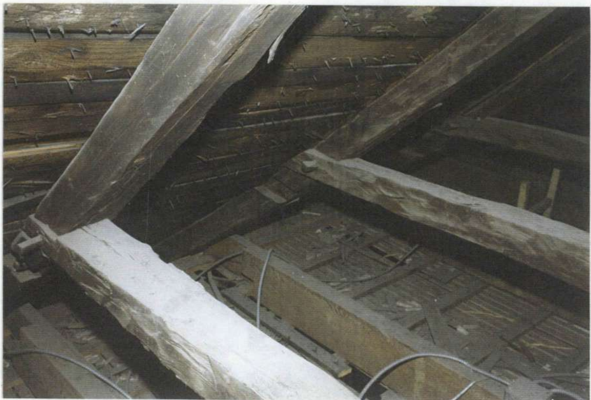
148x. Detail: Attic over space 205. South slope showing that collar ties were raised. Note dovetail notch in rafter below collar tie.
