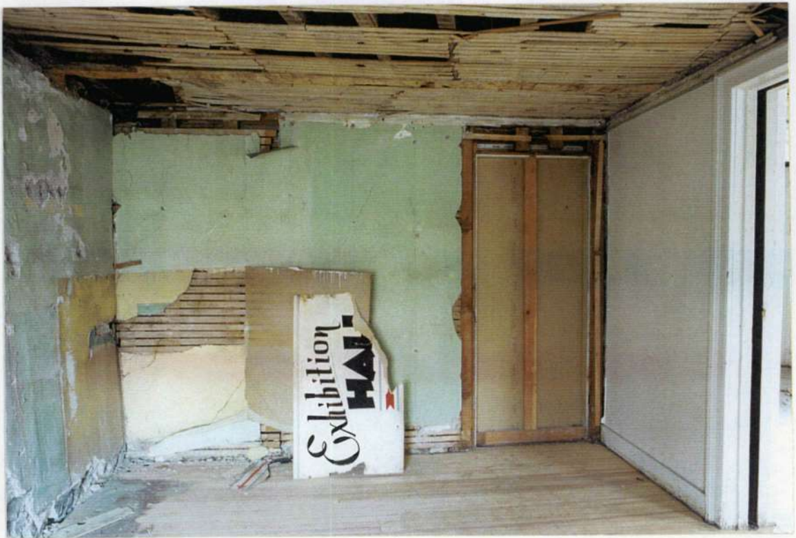
186. Space 109 west wall after removals. Note earlier door (phase five); location of closet on left side at exposed phase four stone wall.
