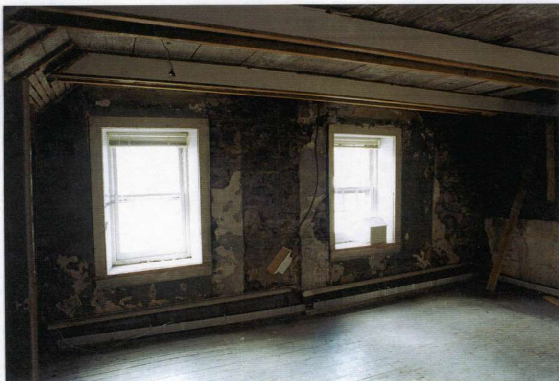
72. Space 201. North wall after removals. Note shadow where removed chimney was located; condition of knee wall juncture and stone gable end; altered collar beams.
