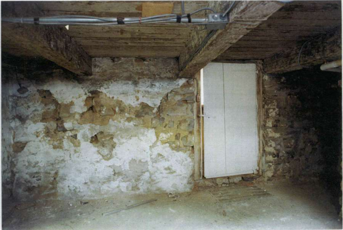
92. Space 002. East cellar rubble stone foundation wall with heavy oak framed Dutch detailed door; Steps up to first floor of phase three.
