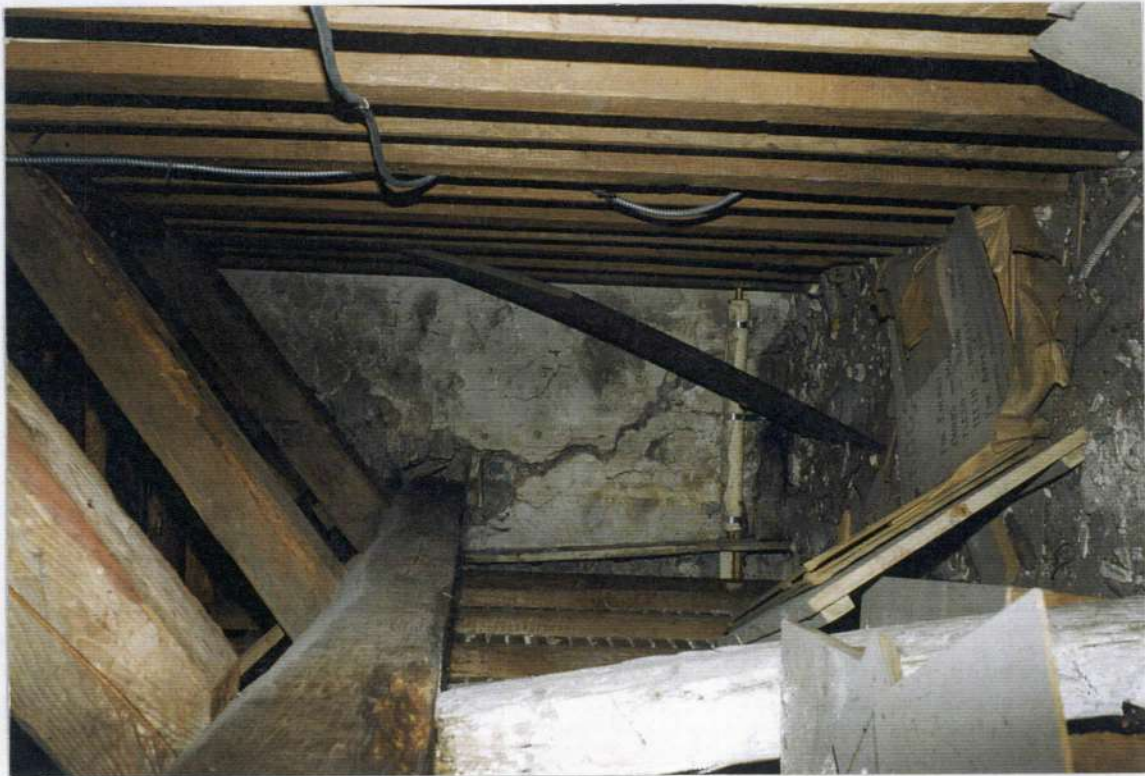
127. Space 204B looking south. Note cracked south stone wall of phase two; horizontal timber supported with vertical (sloping) posts down to top of first second floor beam at wall.
