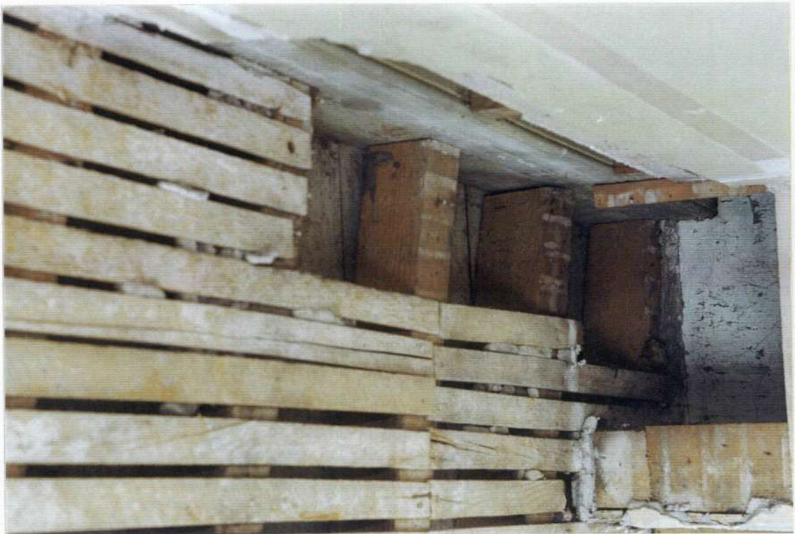
165. Detail: same location at wall looking south. Note early plastered chimney behind and shadow of early plaster where it abuts chimney with paint below. Note that stud framing for built out chimney breast was built under the more original wood lath and plaster ceiling.
