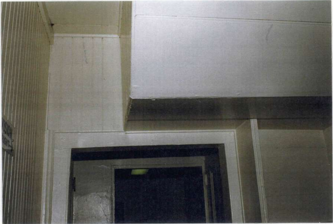
66. Space 202. East wall where rafter and stone wall removed of phase one to make door connection to phase four. Beaded board wall on left is phase five alteration.
