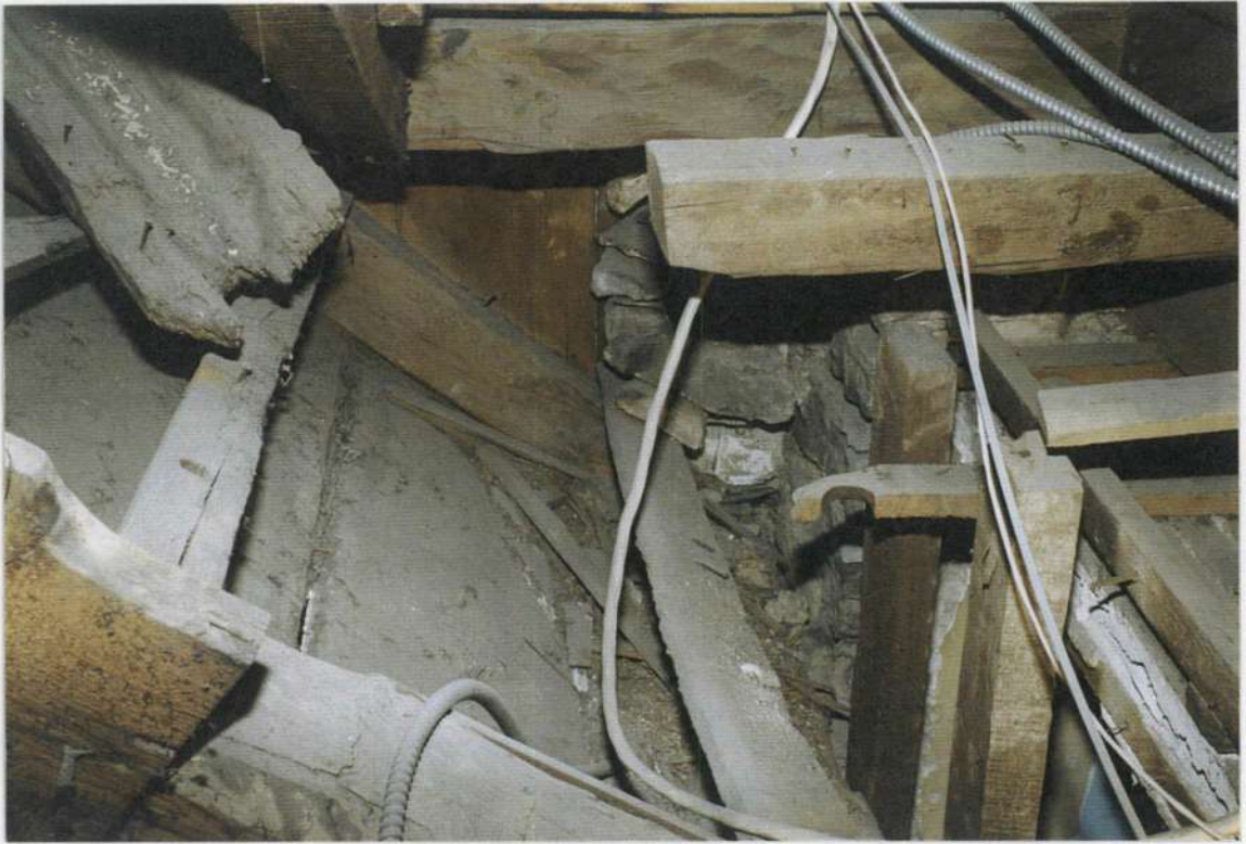
152a. Hand hewn valley gutter of phase four, upper left, built on top of phase one roof. Note end of phase four south stone wall to the right. View looking north.
