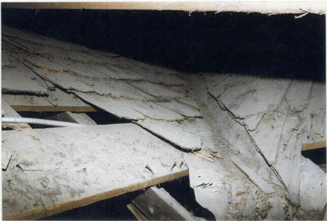
152. Hand hewn valley gutter (covered with tin) at valley intersection of phase three roof to phase two. There is a similar condition where phase four frames into phase one. All roof framing appears to be from 1778 period.
