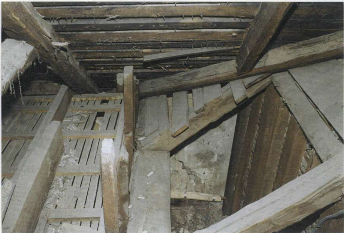
150d. Phase two attic rafter sill plate for wall between phase two and three looking south. Note valley rafter of phase three built on top of phase two rafters to the right.
