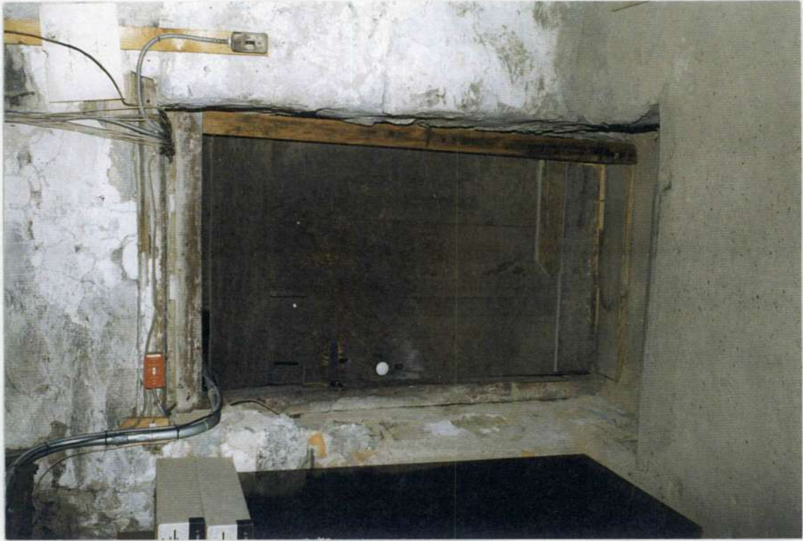
154. Cellar door between spaces 001 and 003 as seen from space 001. Door frame mortise and tenon pegged framed.
