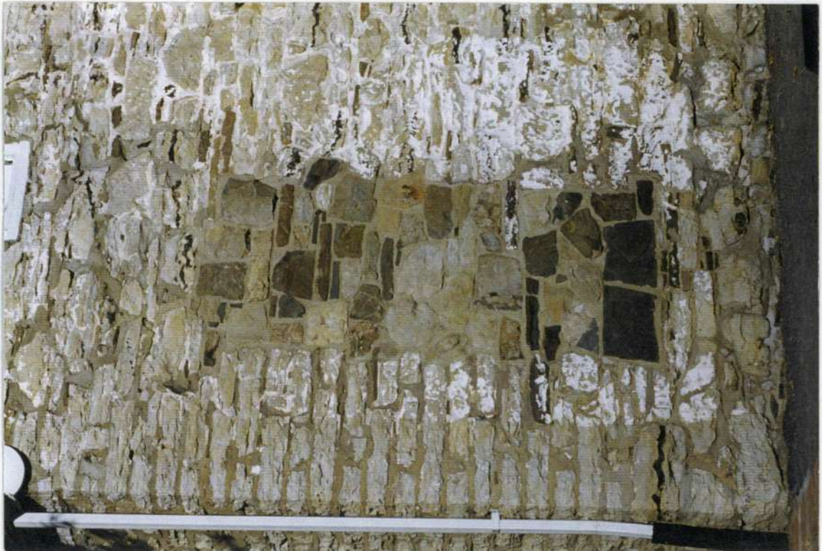
35. South phase two wall where door removed during phase five. This end of building had one story wood framed addition in late 1800s.
