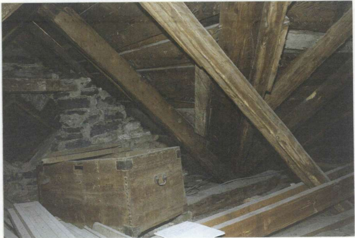
91b. Attic of phase one looking at phase four hand-hewn valley gutter and rafter built on top of phase one rafters. Note stone infill to north gable end.
