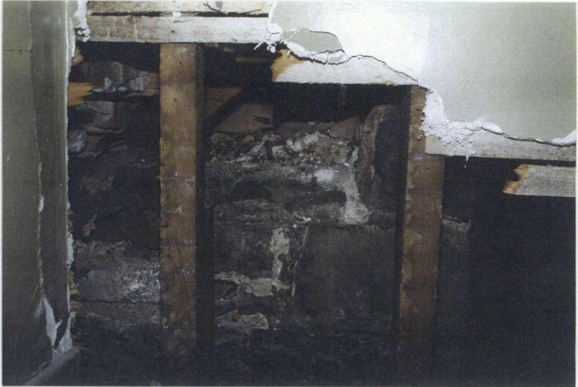
153a. Southeast corner of phase four stone wall added to east wall of phase three looking west, as seen from phase five. Note end of south roof sill plate at corner and brick end wall of phase five.
