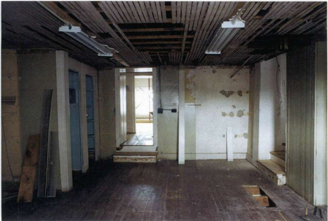
140. Space 205 north wall after removals. Note beaded board walls; lath and plaster ceiling which was installed phase five.
