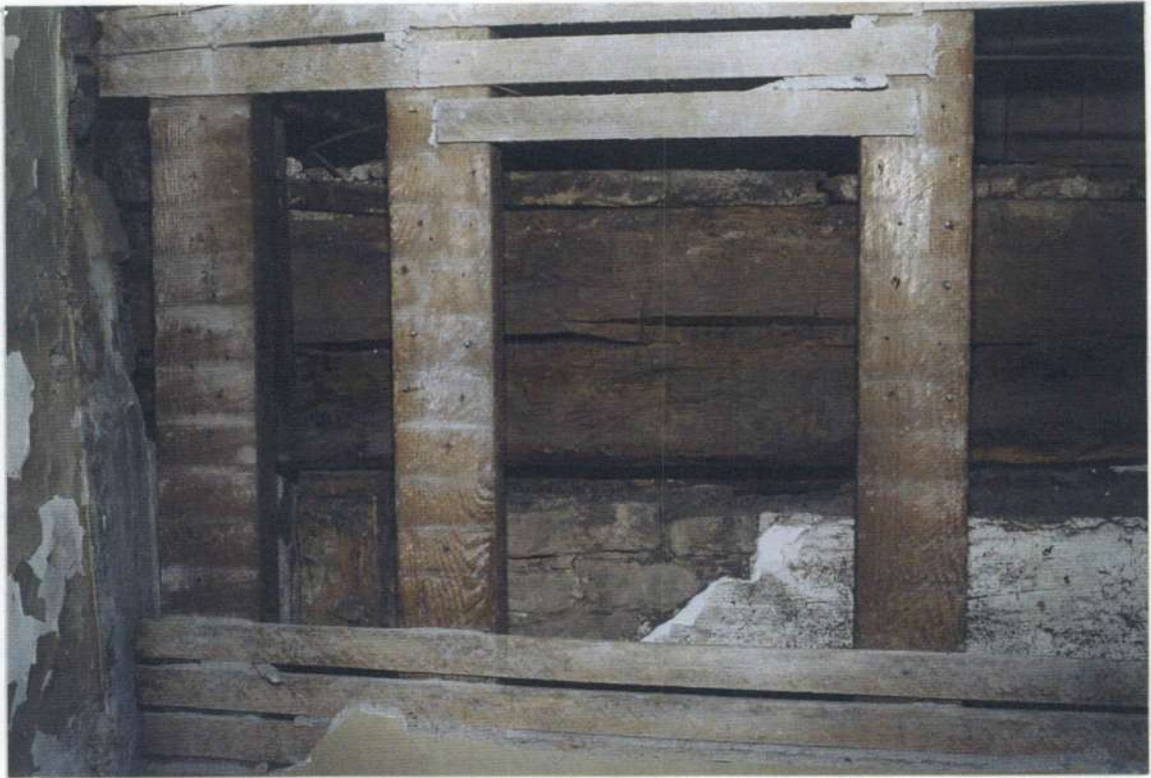
148a. Space 205. West wall after removals. Second floor beam and floor planks of phase two at south end wall with hand-hewn post and brick infill, stucco finish.
