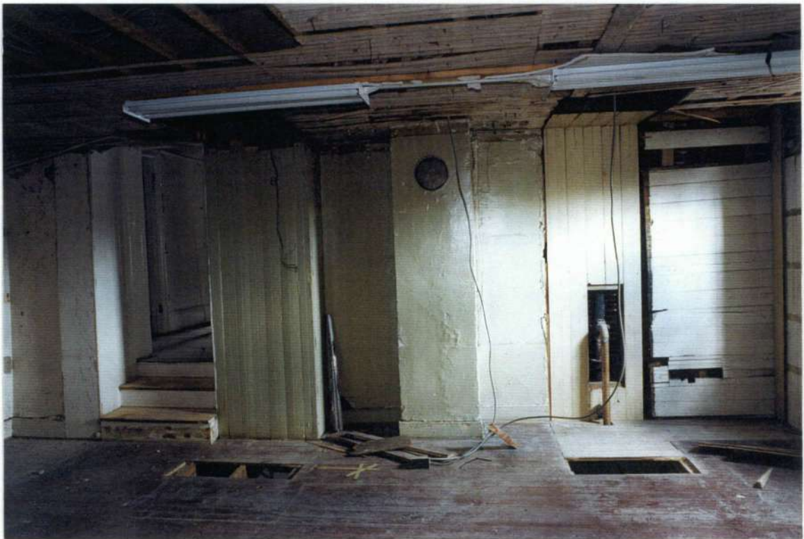
148. Space 205 east wall after removals. Note plastered chimney and stove pipe connection.
