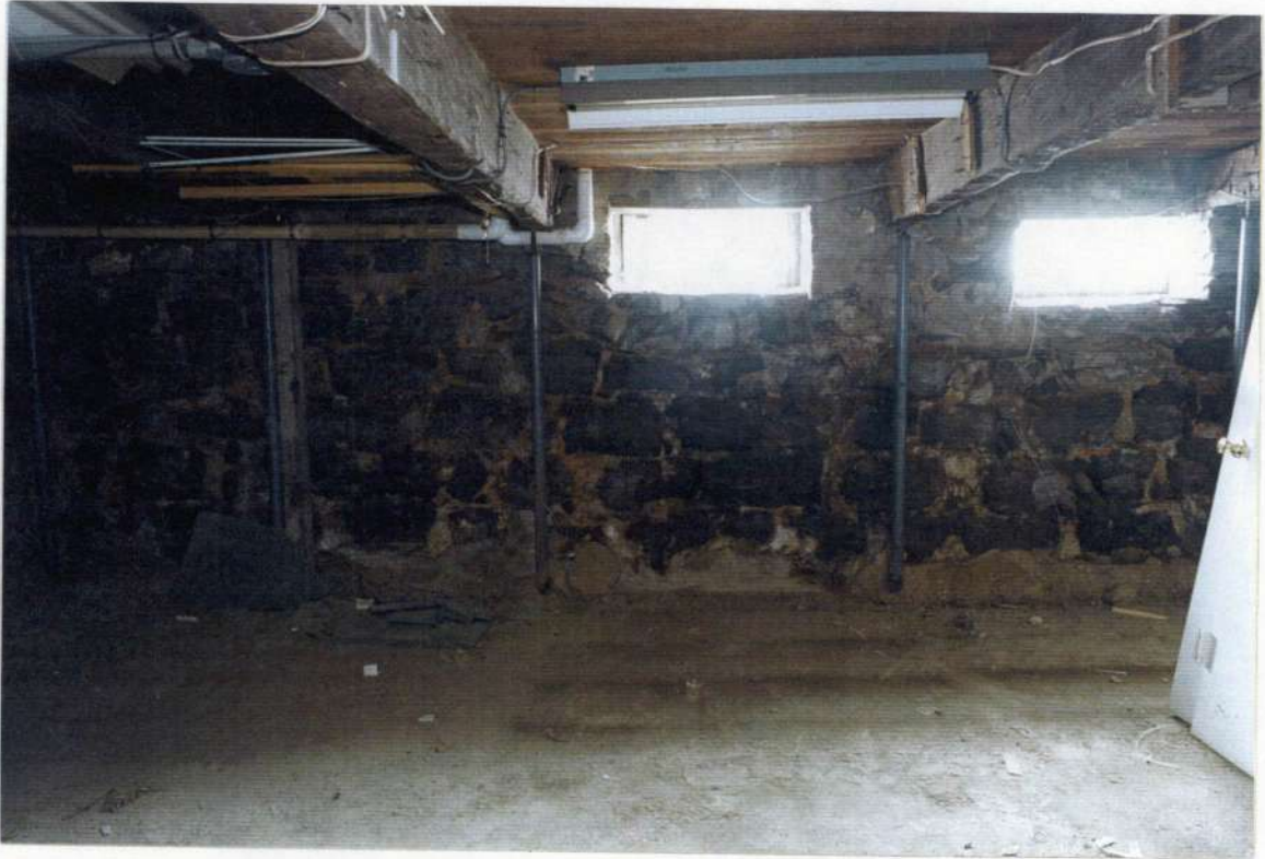
42. Space 001 west wall. Typical rubble foundation wall requiring repointing.
