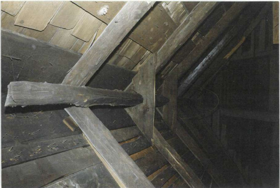
148w. Detail: Attic over space 205. Phase three ridge detail supporting jack rafters over roof connection between phase two and three. This ridge detail is similar between the connections of phase one and four.
