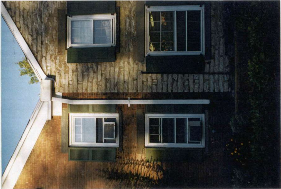
30. Joint between phase four stone and phase five brick addition. Note bluestone lintels and sills of phase five added over tops of phase four east façade windows; wider first floor window added phase five. Note wood shutters and plastic shutters of phase five.
