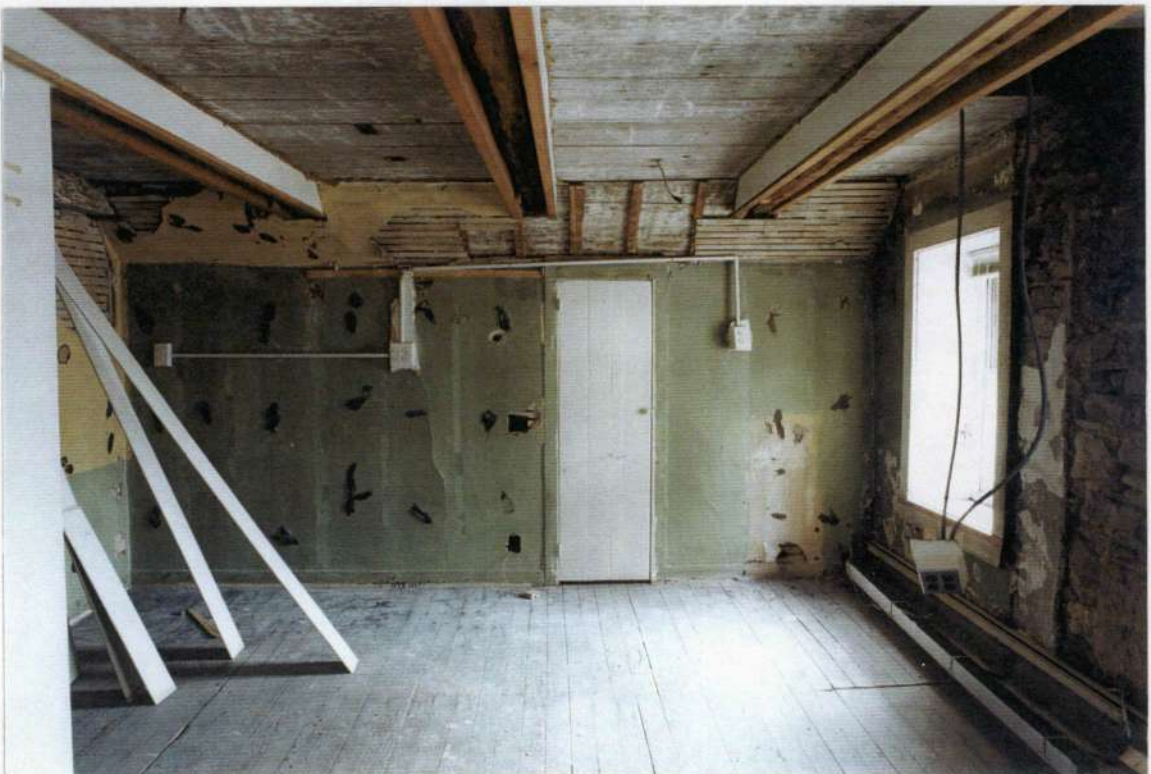
76. Space 201. West wall after removals. Note plaster end wall (a similar wall was removed on east side of room); plaster and wood lath added over sloped wood plank ceiling.
