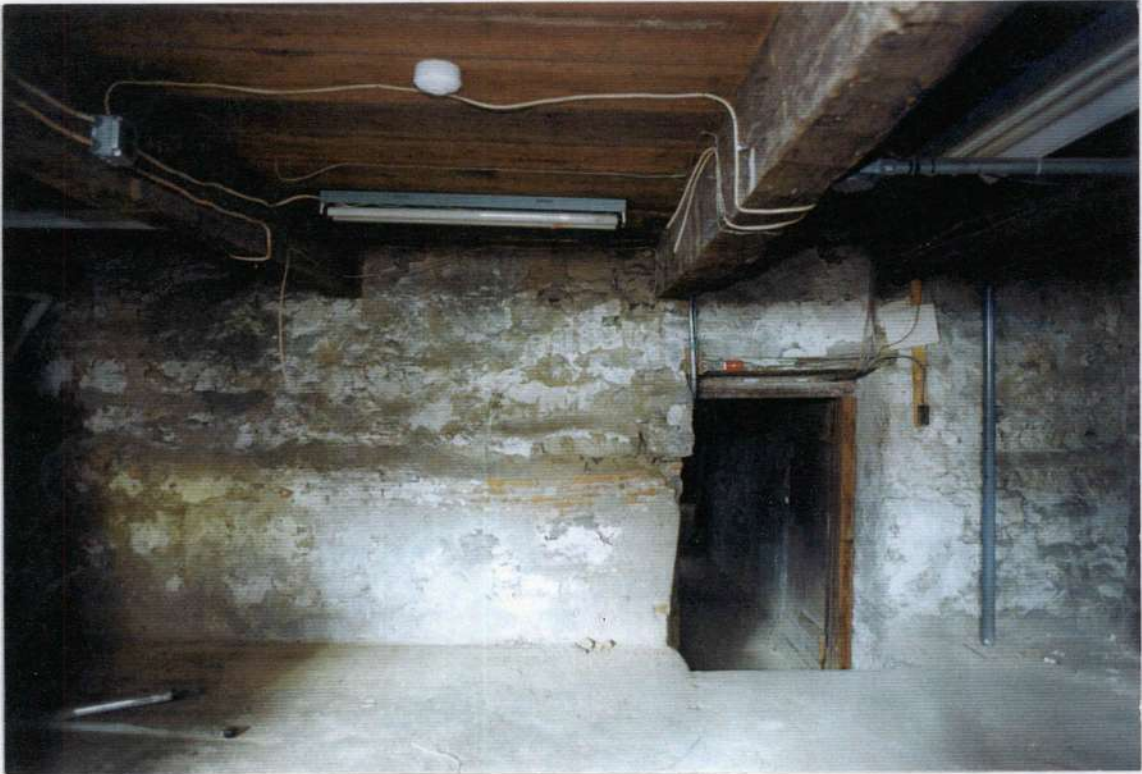
40. Space 001 east wall. Possible early arched brick Dutch fireplace first floor hearth support detail. Note wide board floor planks and hand hewn beams.
