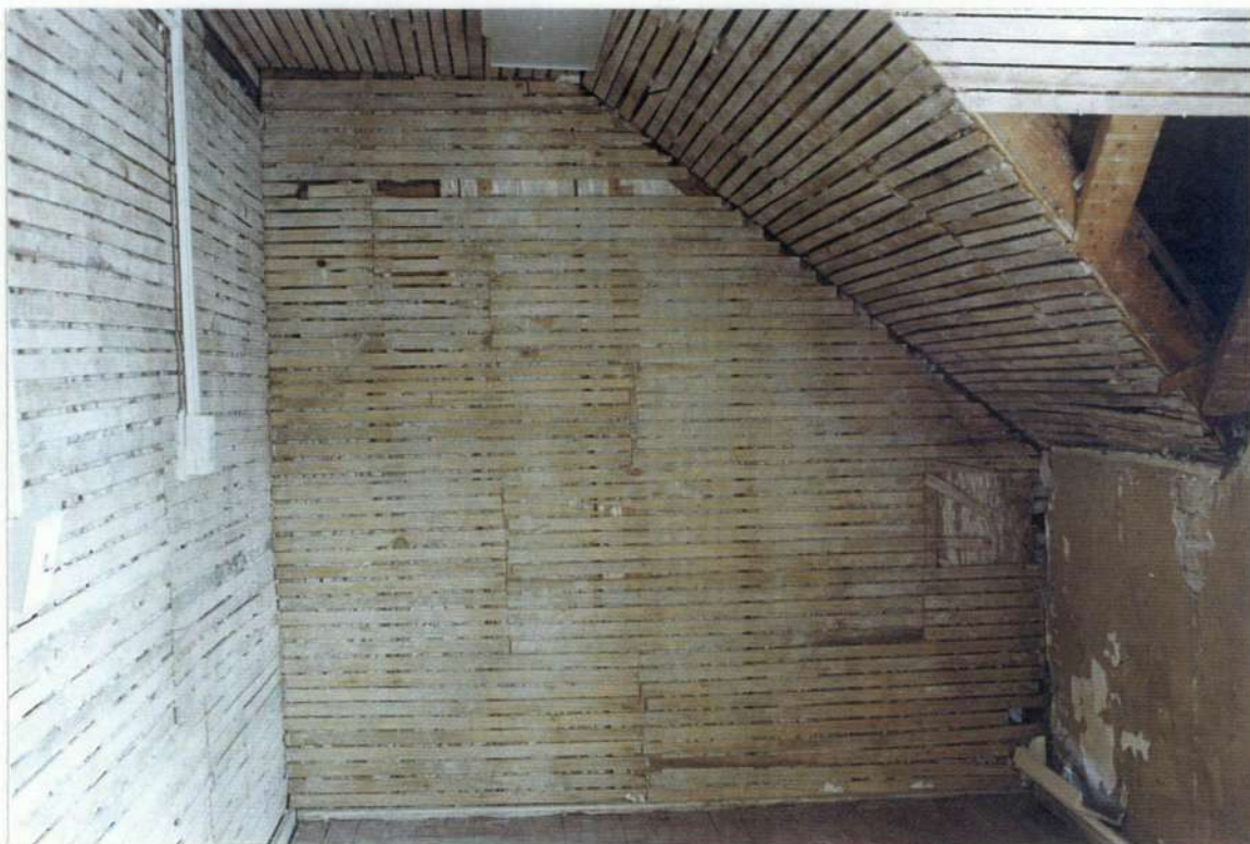
90. Space 203 south wall. Ca. 1850s wood lath and plaster over earlier vertical plank wall. Note valley detail of roof and new gable.
