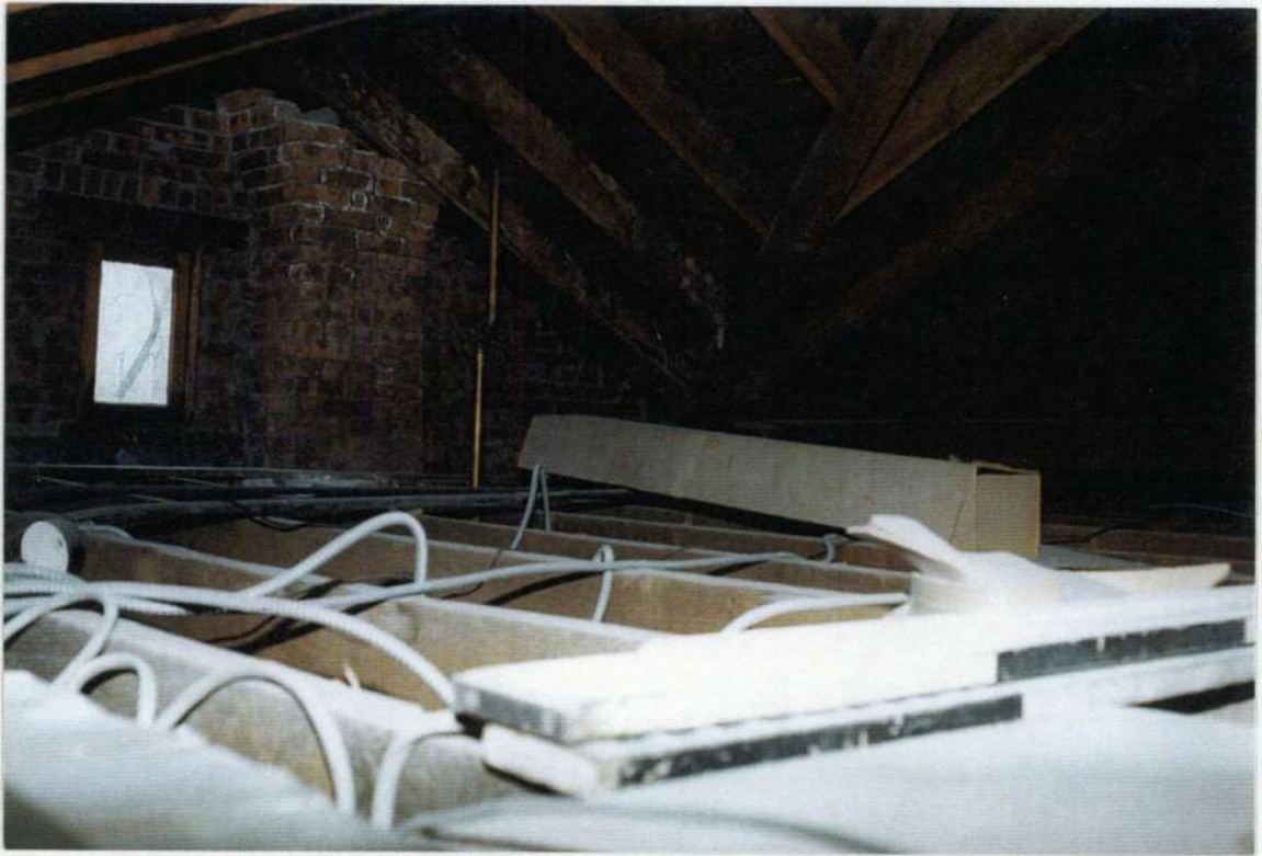
255. Attic over space 212 looking east. Note abandoned brick chimney.
