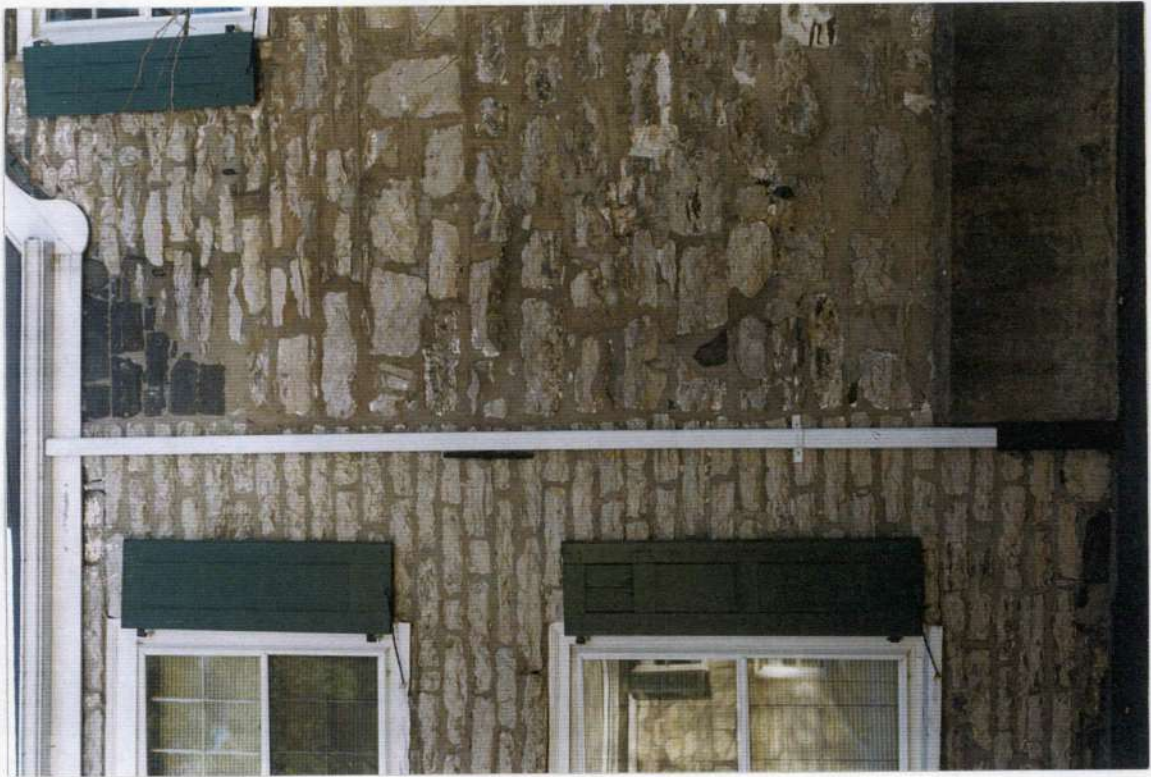
26. Joint between phase one and four. Note change in stone pattern, concrete base reinforcement of phase one, iron beam anchor at second floor level.
