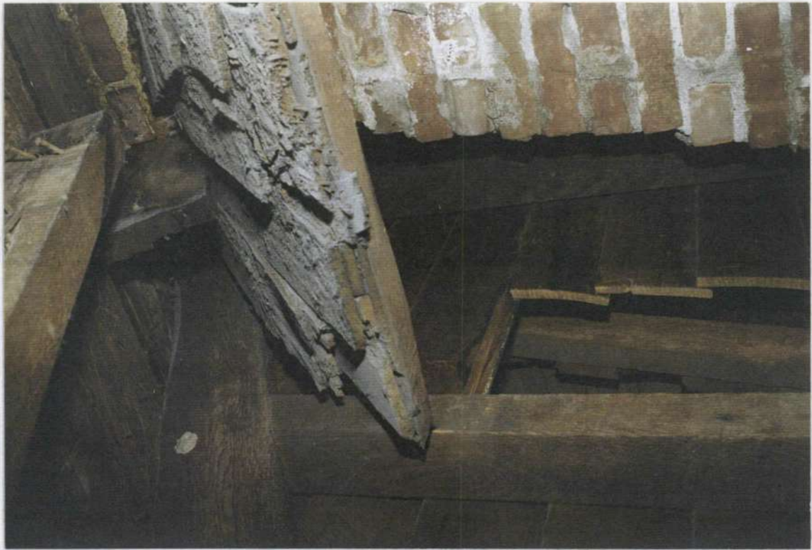
148q. Attic over space 205 at east clapboard gable end. Original phase three roof and framing at chimney and later phase four upper roof.
