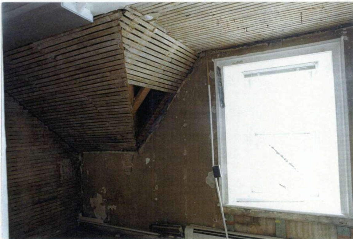
89. Space 203 west wall. Note plastered exterior stone wall; higher window of ca. 1850s ceiling in this space was raised above the wood plank ceiling of other phase one spaces. This space would not have had a window before this period.
