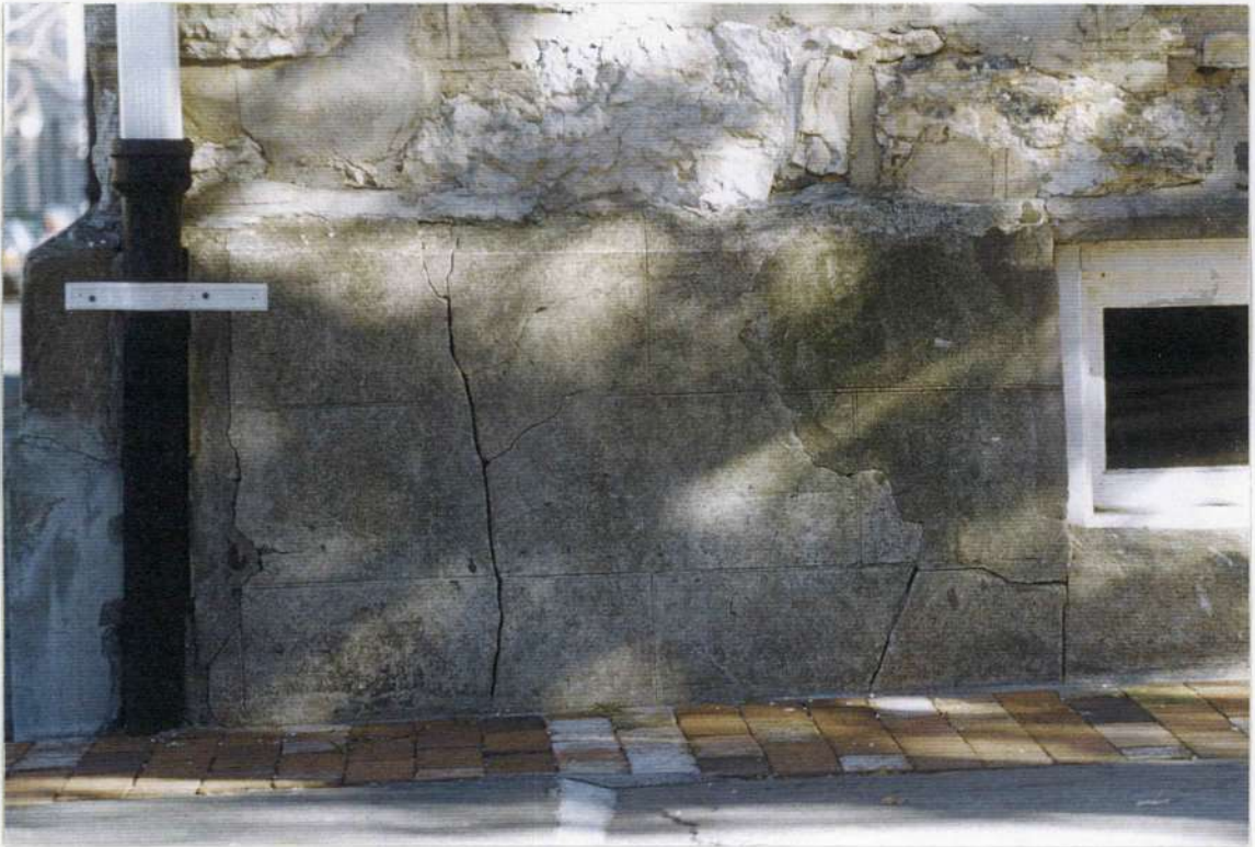
22. Detail: Applied concrete base to lower phase one wall at corner of Crown and John Streets.
