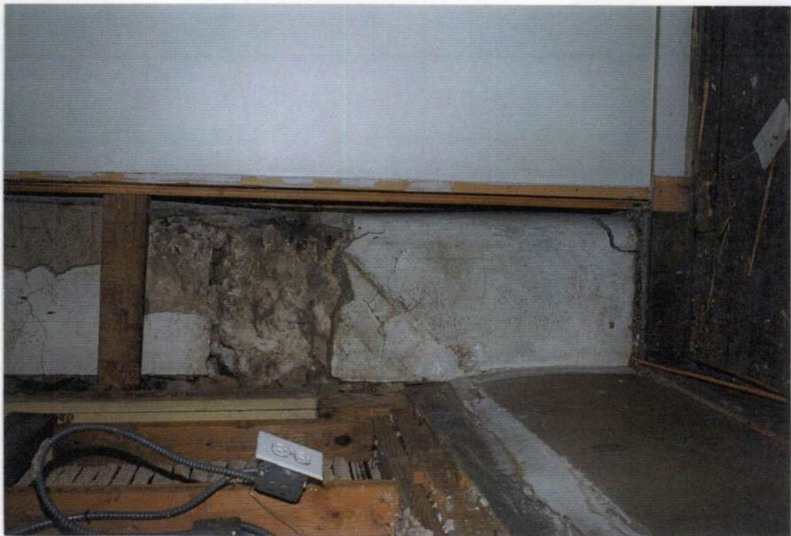
137. Detail: exposed plastered exterior corner of phase one showing shadow of stair stringer up in corner. Note rounded lower exterior wall corner of phase one stone wall.
