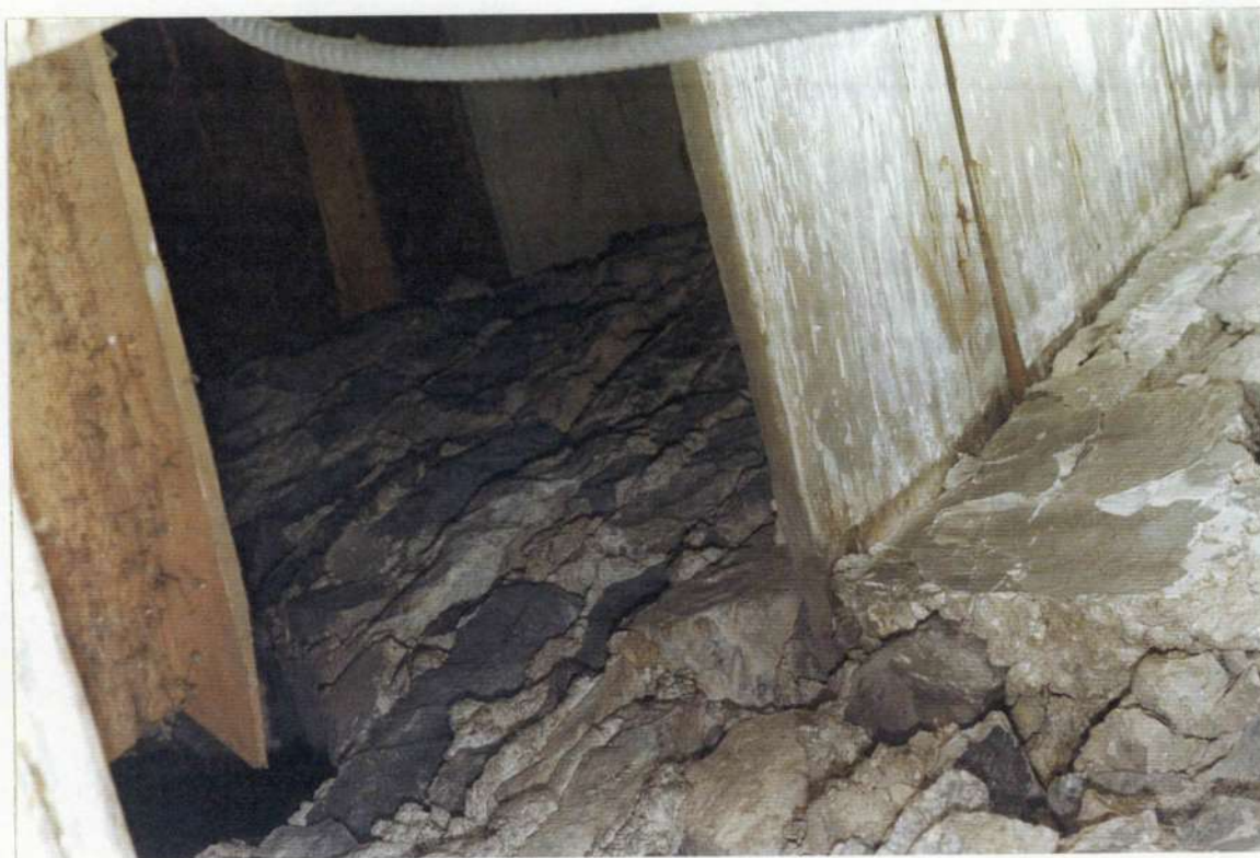
82. Detail: Space 201 north wall: early ceiling plank adjacent to removed chimney opening showing that stone gable end wall was built on top of planks at window height. Earlier wood framed upper gable end wall was removed and replaced with stone ca. 1850s.
