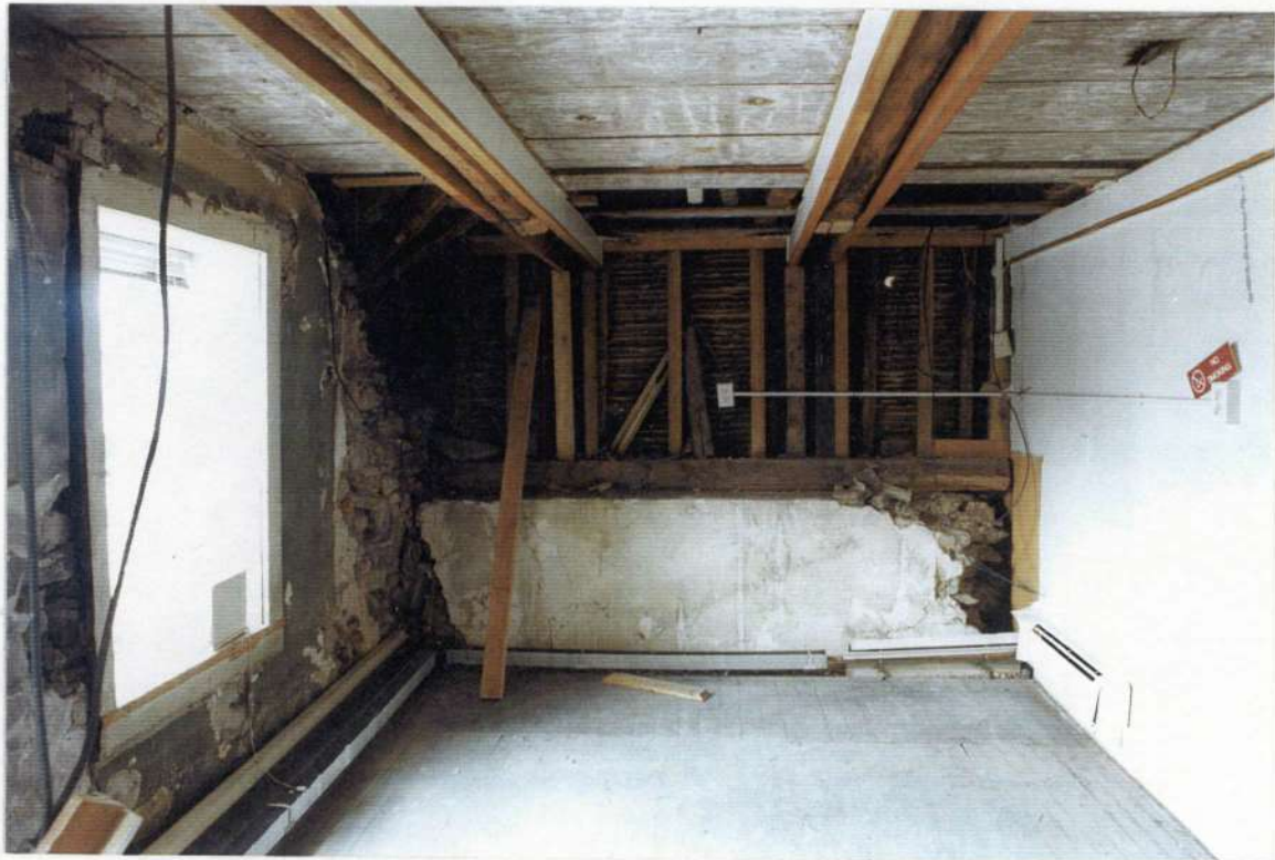
70. Space 201 after removals. Note stone knee wall; upper phase four stud and plaster wall; and phase five altered collar beams and roof rafters below wood plank garret loft floor.
