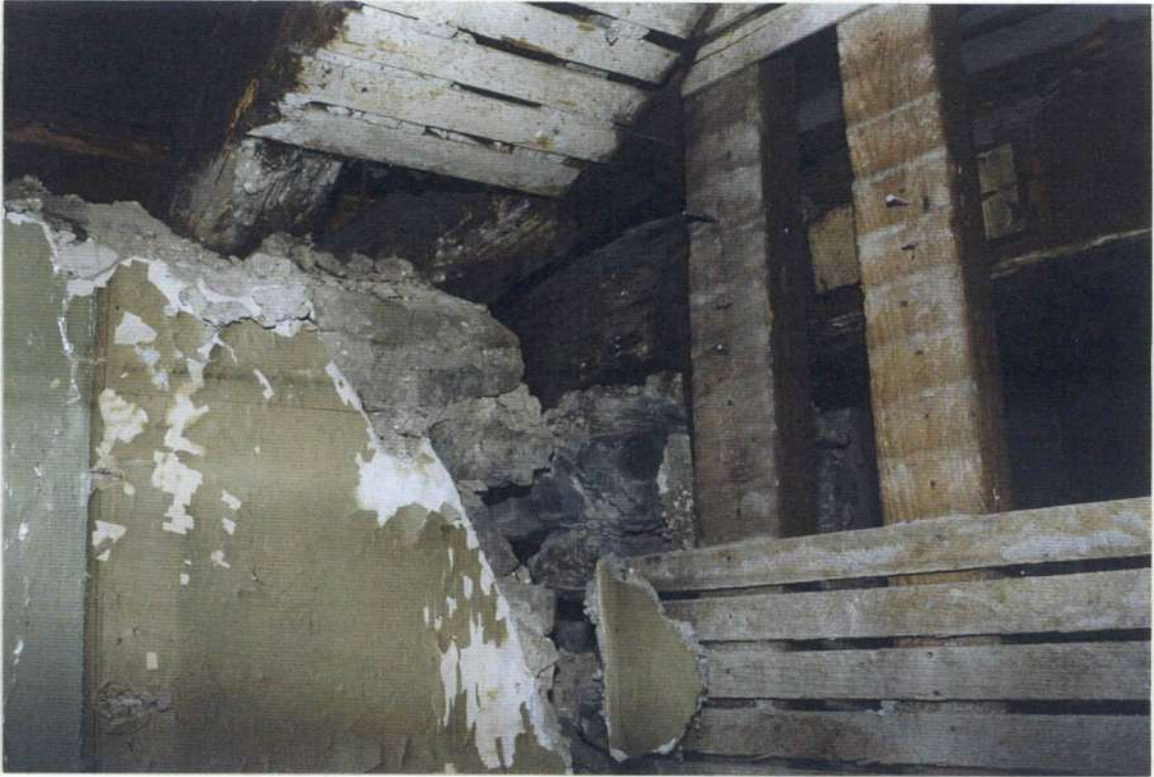
148c. Space 205. Southwest corner. Phase two roof sill plate into stone wall; phase three roof framing at corner.
