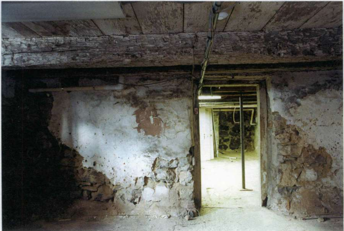
93. Space 002 north wall (exterior side of south phase one wall) with heavy oak door frame to space 001. Note early plaster on stone wall with paint finishes; wide board plank floor and hand hewn beams above.
