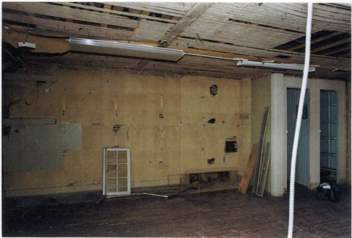
143. Space 205. West wall after removals. Closets and door to stair down built as part of phase five. This space had a tin ceiling over the earlier plaster ceiling.
