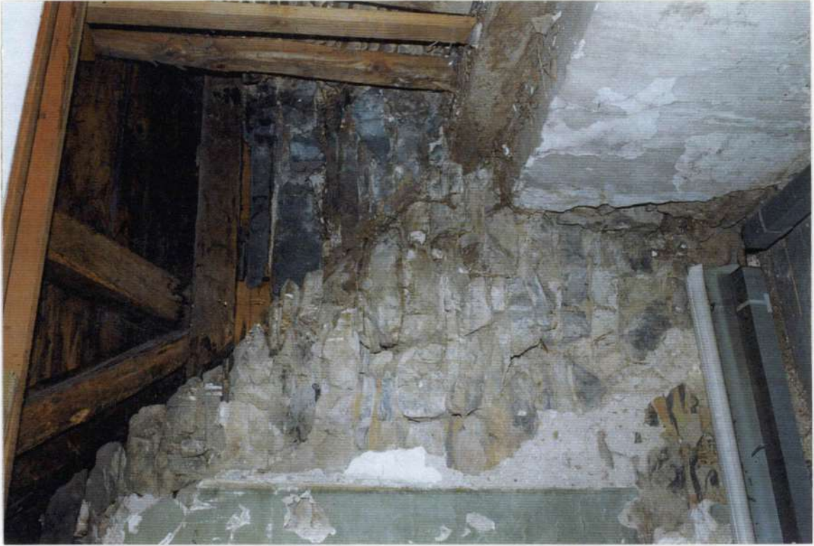
73. Detail: northeast corner of stone wall missing.
