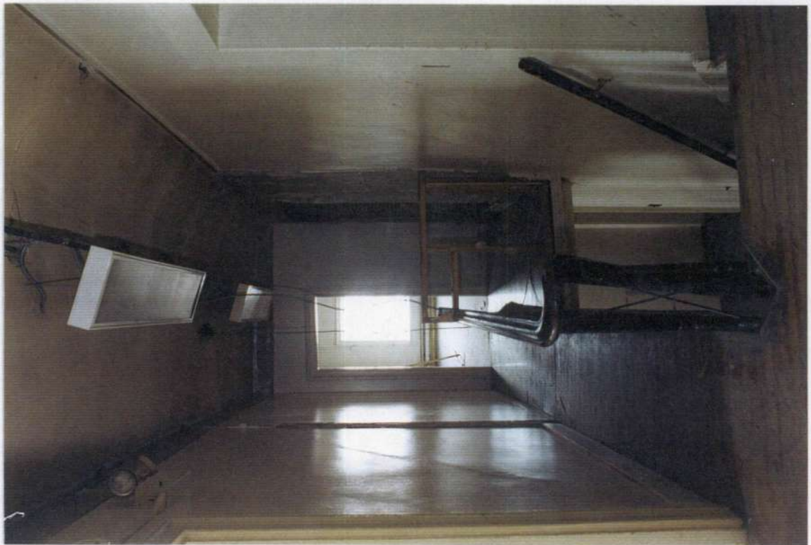
194. Space 210 looking east after removals. Note space 209 wall removed; hall wall on left built to underside of earlier plaster ceiling. This wall is built as thin stud wall.
