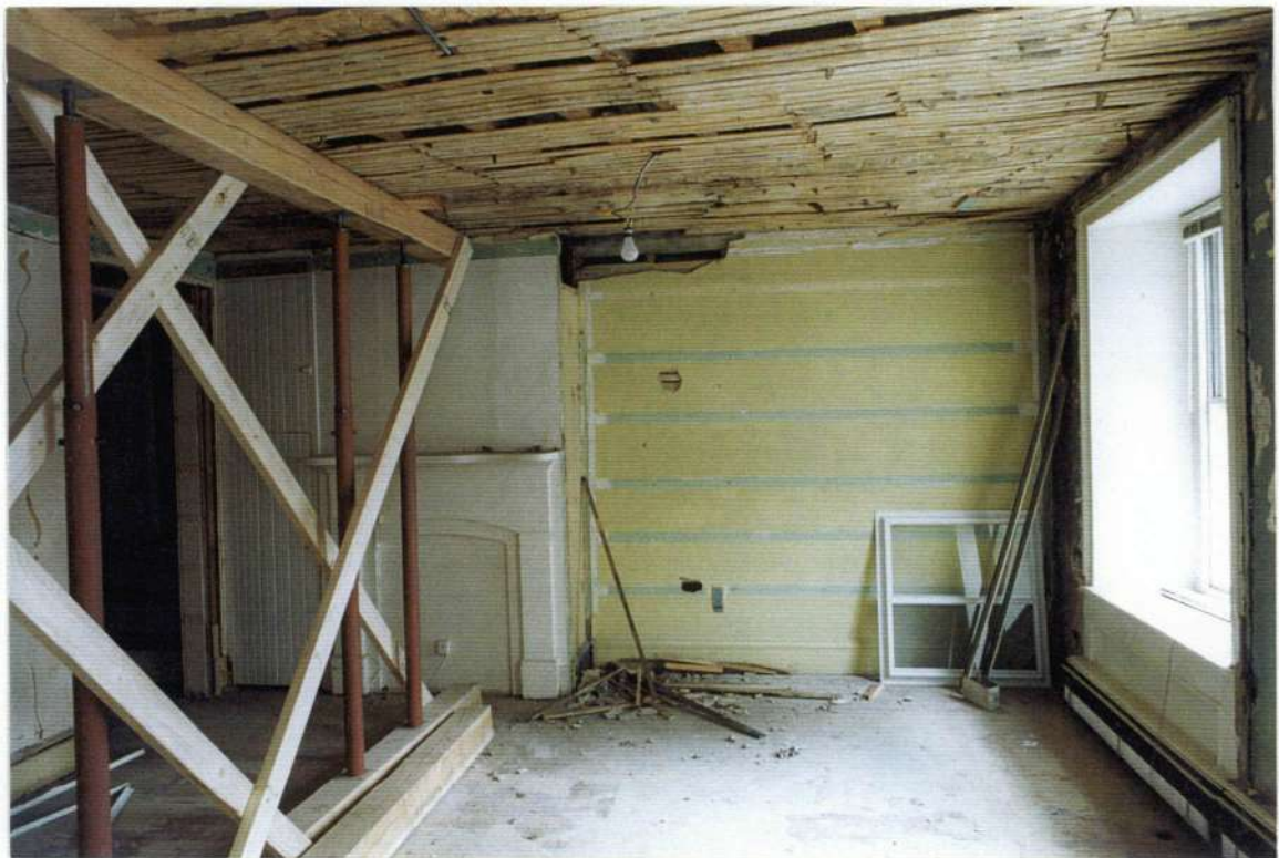
163. Space 105 west wall after removals. Note emergency roof shoring from above; lath and plaster ceiling with original beam bottoms cut off.
