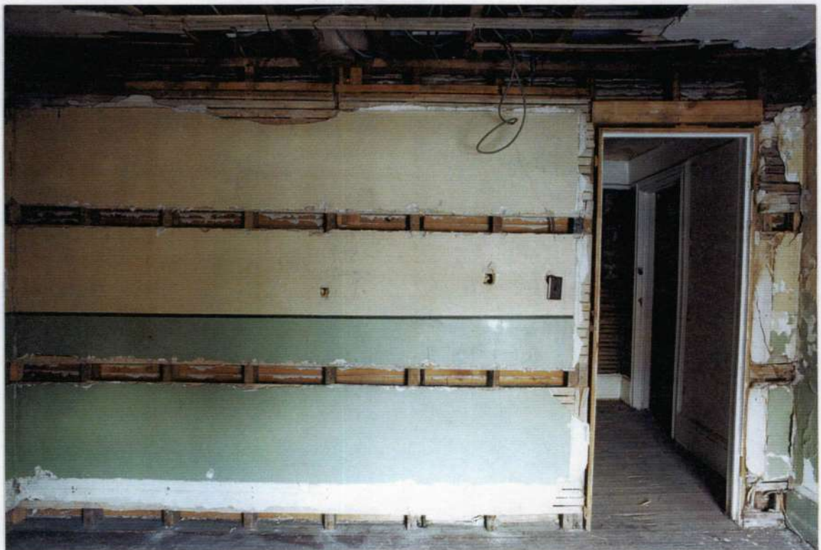
239. Space 212 west wall after removals. Note strips (bands in wood lath wall) are from nailers used to attach recent wood paneling.
