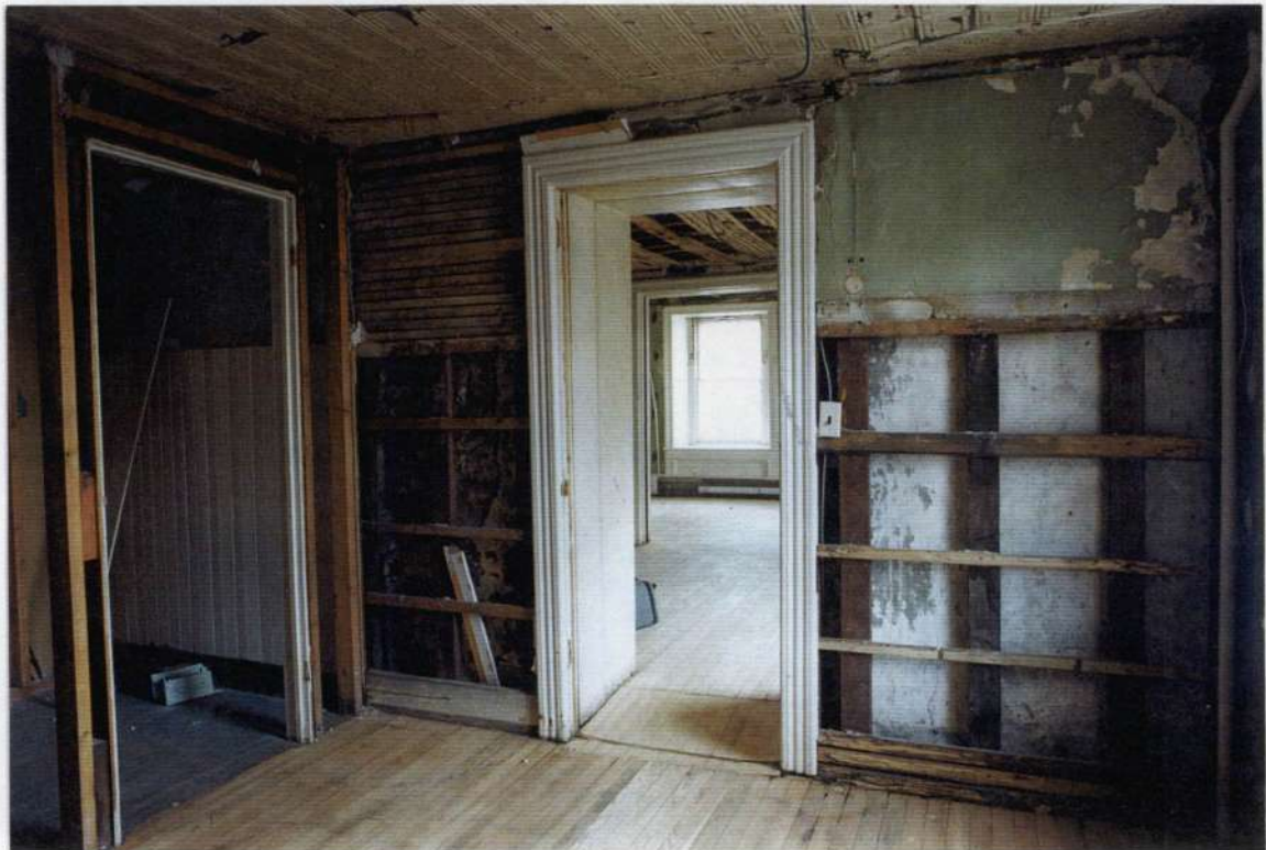
226. Space 112 north wall after removals. Note exposed exterior wall of phase four behind framing of phase five wainscoting. Note tin ceiling.
