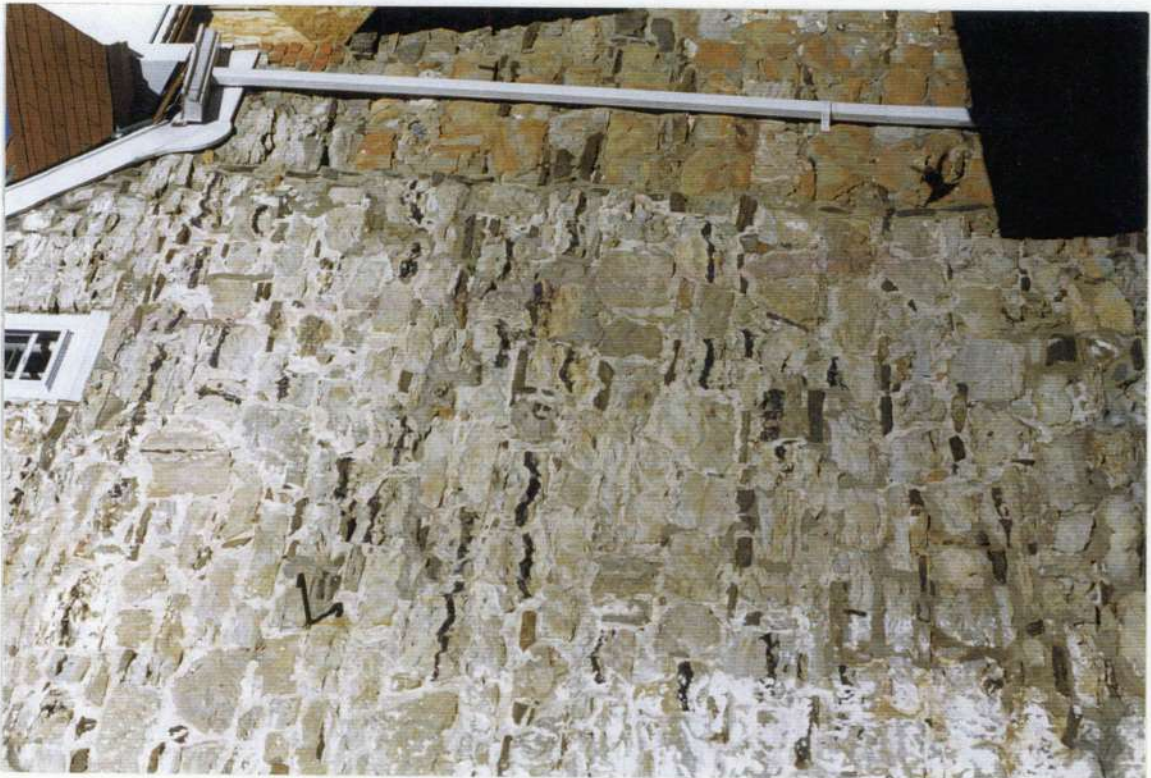
33. Joint between phase two addition and phase three (phase five stone wall). Note whitewash on phase two wall.
