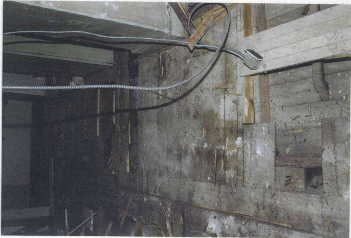
148j. Space 205 east wall looking north. Area where stone wall and fireplace of phase three removed in phase five.
