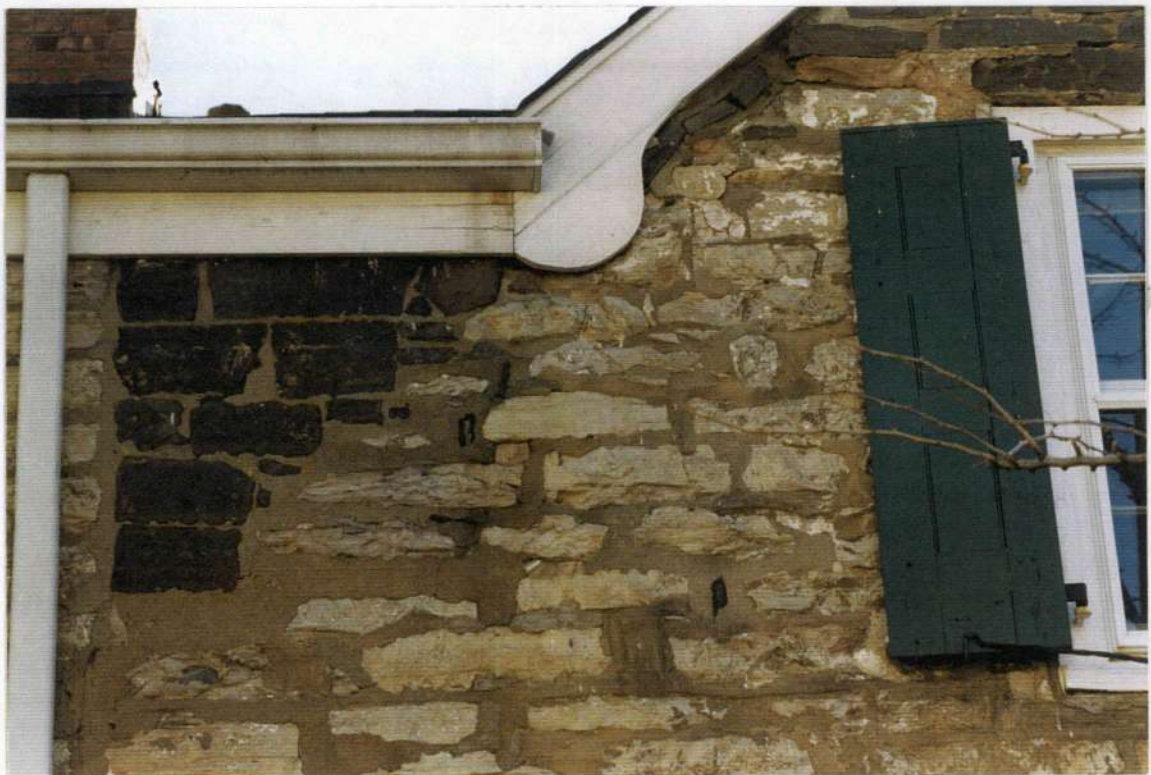
27. Detail: ca. 1850s stone infill where phase one roof framing line was before phase four addition was attached.
