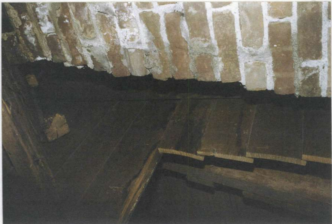
148r. Attic over space 205 at east clapboard gable end. Underside of original phase three roof and hand hewn beam framing. Note cut-off rafter end.
