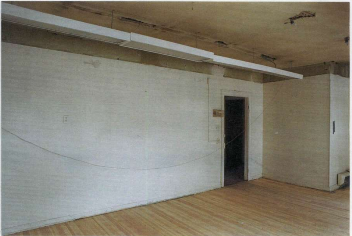
197. Space 206 south wall after removals. Note ceiling height above recent hung ceiling.
