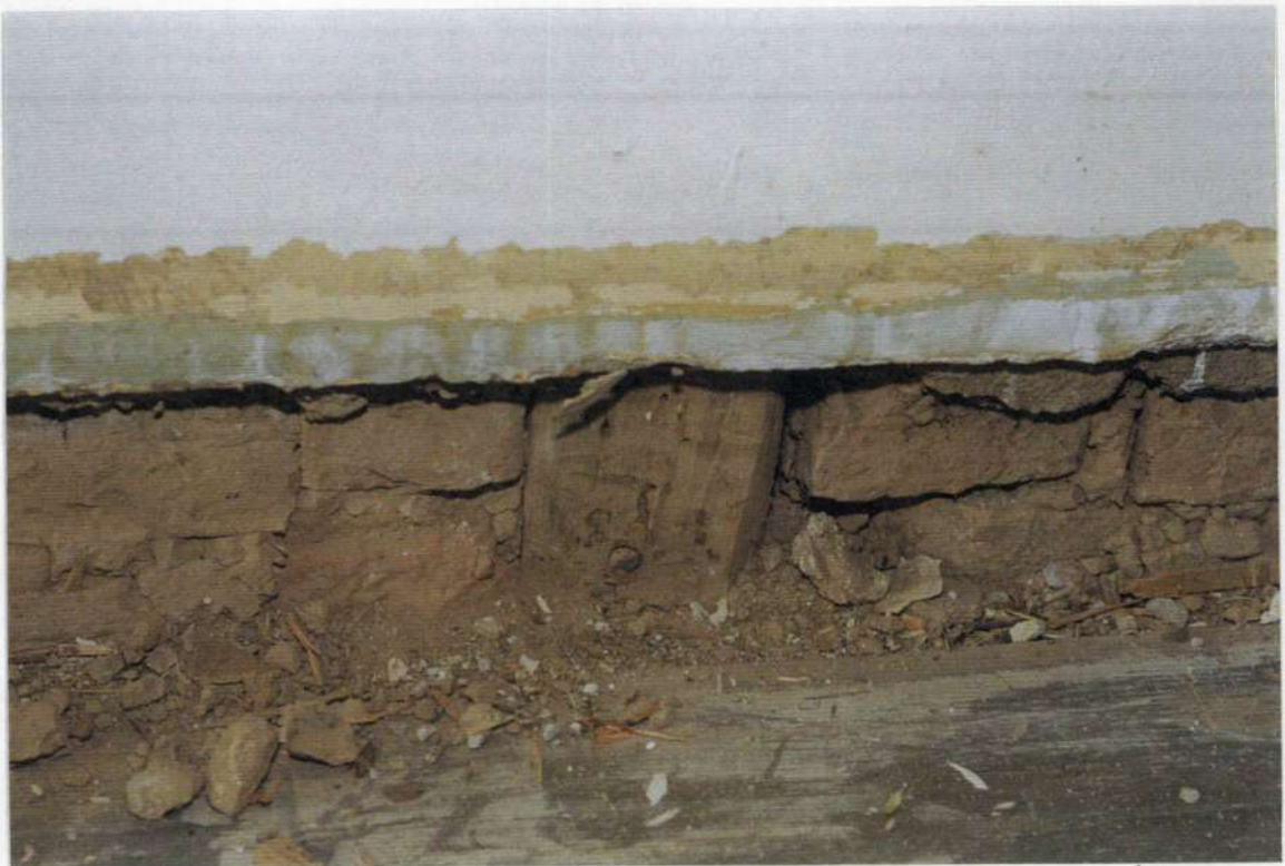
61. Space 102. North wall, east end behind baseboard. Brick infill between hand hewn stud. Similar detail possibly at west end of wall.
