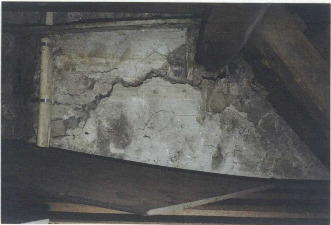
148f. Space 204B. Southeast corner of phase two roof sill plate and stone wall. Note side of wood beam in stone wall at floor, possible phase three wood framing.
