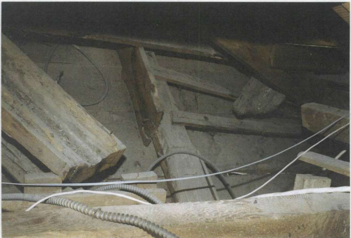
152b. Hand hewn valley gutters of phase four (right) and phase three (left) built on top of phase one and two roofs respectively. The sloped rafter in the center of the photo is the last gable end rafter of the south end of phase one.
