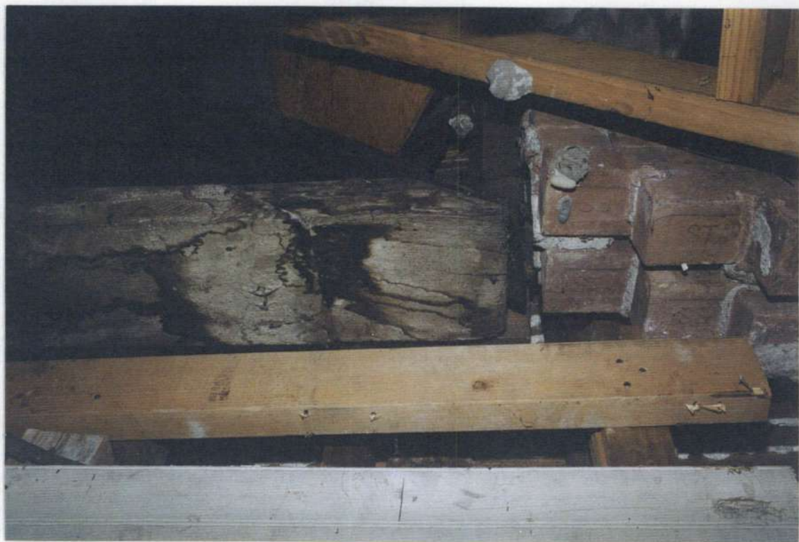
148n. Space 205. Top of stone wall as seen in photo above. Note underside of sill plate installed with phase four stone wall, end of original phase three hand-hewn rafter and phase five brick wall.
