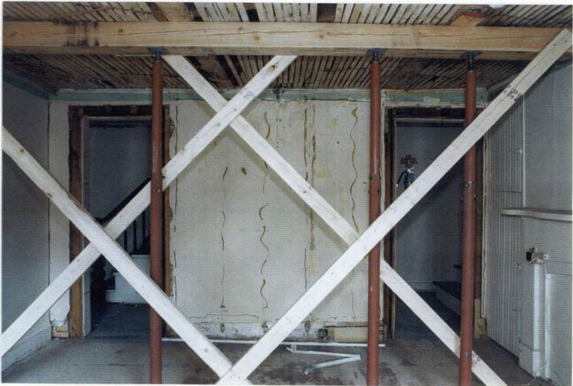
167. Space 105 south wall after removals. Note two earlier (phase five) doors covered. This wall was also built below an earlier plaster ceiling and after the beam bottoms were cut off.
