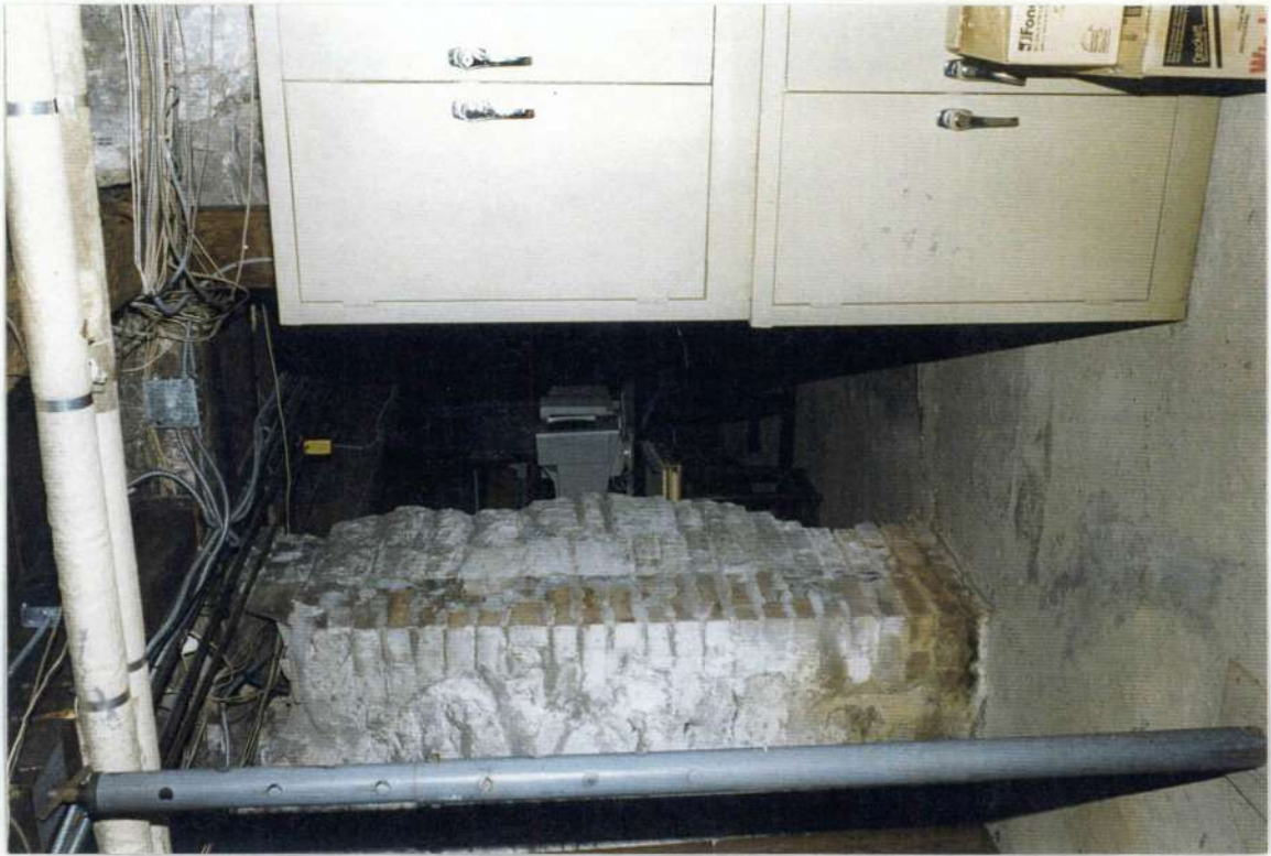
156. Opening in phase four foundation wall from space 003 to phase five. Note bricked opening and rough exterior side foundation wall of phase four.
