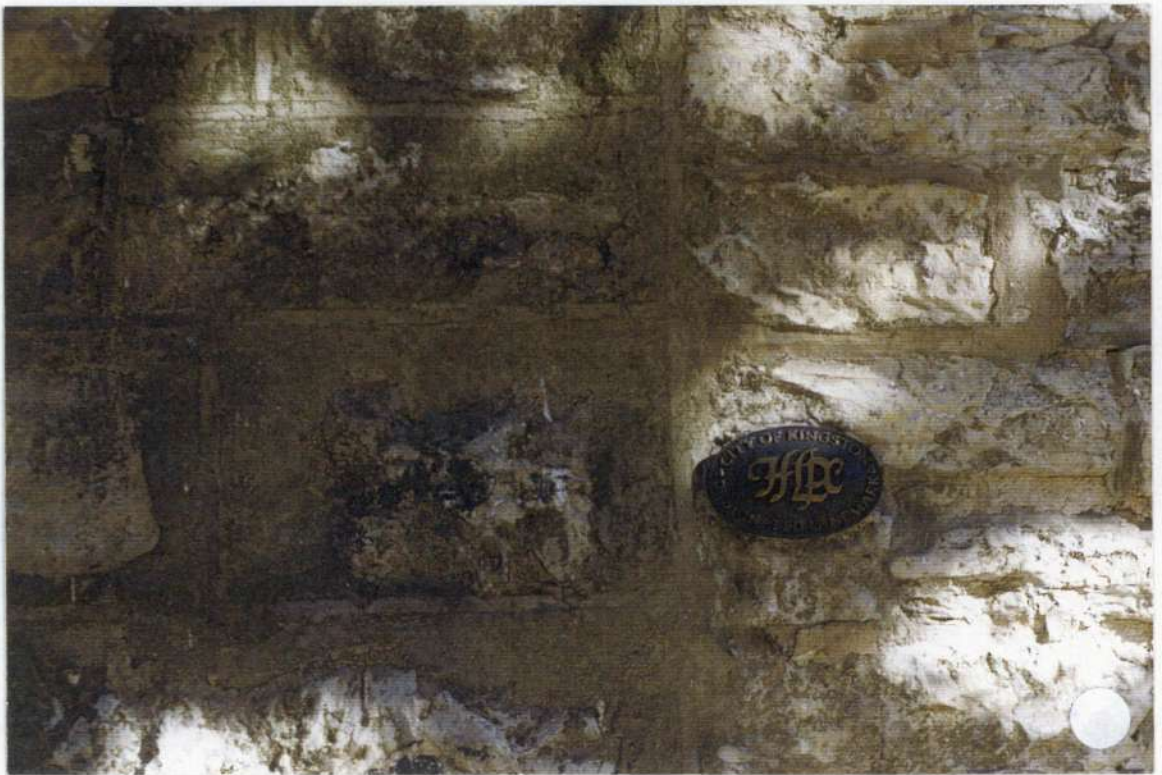
21. Detail: Note stone coursing in jointwork of rubble stone of phase one made to match phase two and four.
