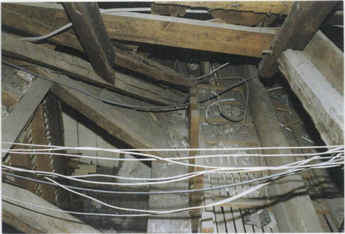
150c. Phase two attic rafter sill plate for wall between phase two and three looking north. Note valley rafters of phase four, to the left, built on top of phase two rafters. Valley gutter behind valley rafter.
