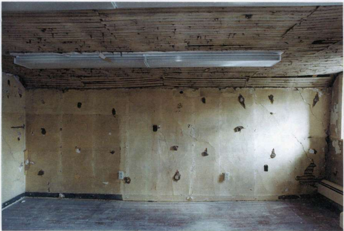
117. Space 204. East wall after removals. Note wood lath and plaster ceiling (below collar ties).
