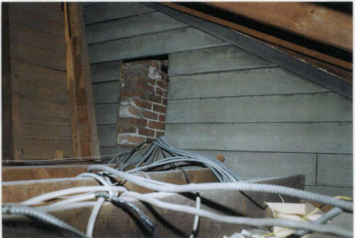
153. East wood framed exterior clapboard gable ended roof of phase three as seen from phase five attic.
