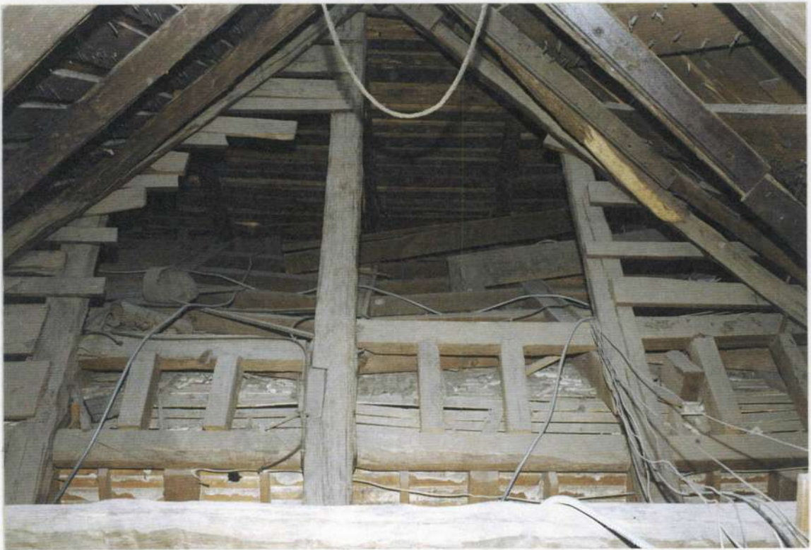
148v. Attic over space 205 looking west at phase two roof rafters. Both attics are open into each other.
