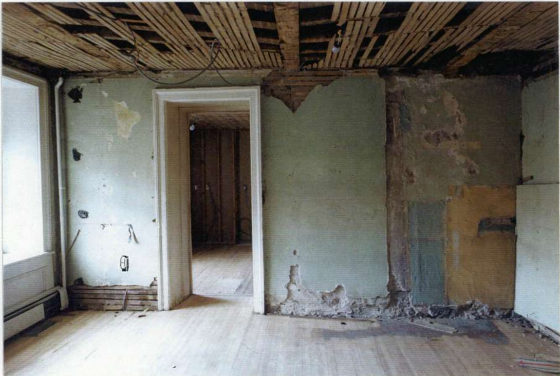
188. Space 109 south wall after removals. Note wood lath and plaster ceiling, cut beams, exposed interior side of phase four stone wall plastered (right side), and wood lath and plaster over stone wall (left side) indicating possible stone wall deterioration.
