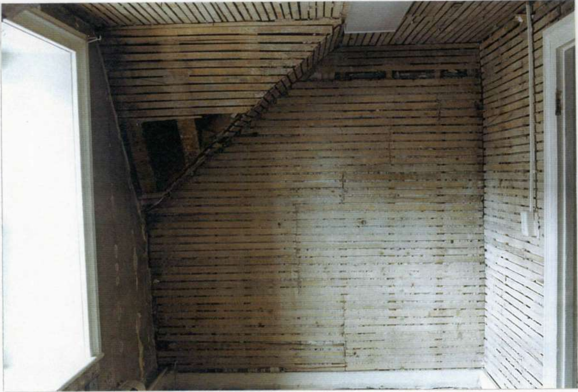
87. Space 203 north wall. Ca. 1850s wood lath and plaster over earlier vertical plank wall. Note valley detail of roof and new gable.
