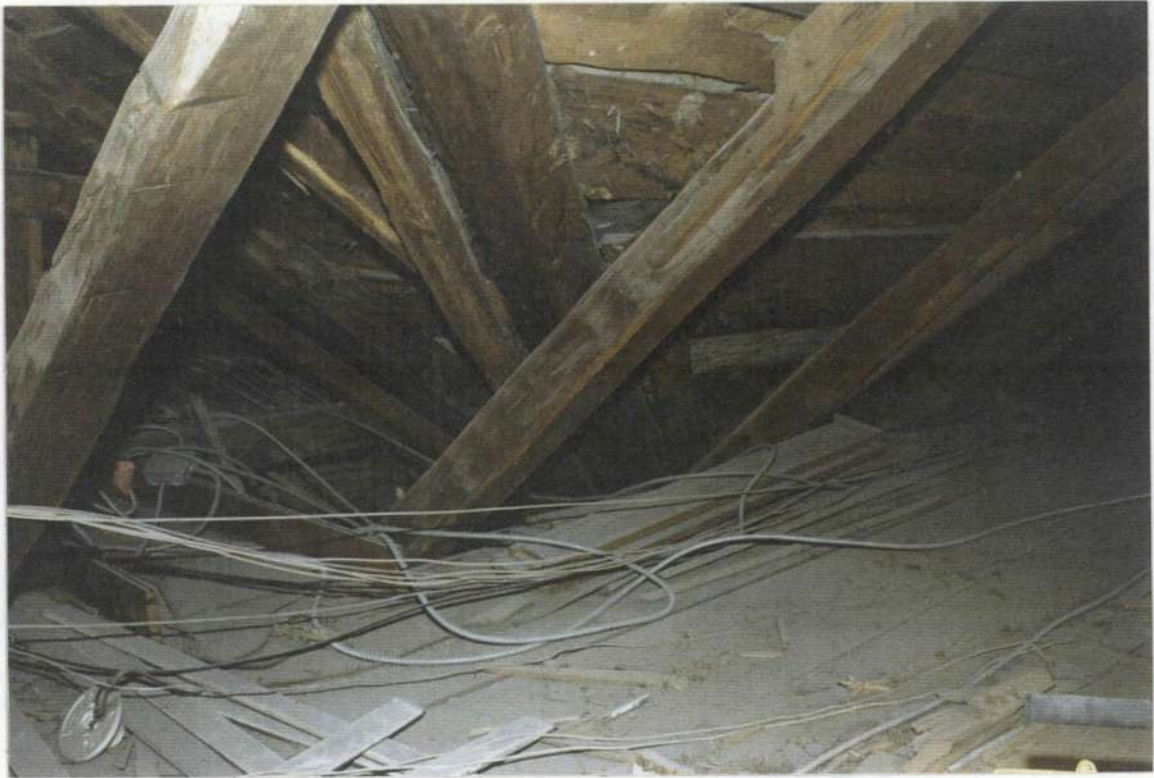
91a. Attic of phase one looking at phase four hand-hewn valley gutter and rafter built on top of phase one rafters.
