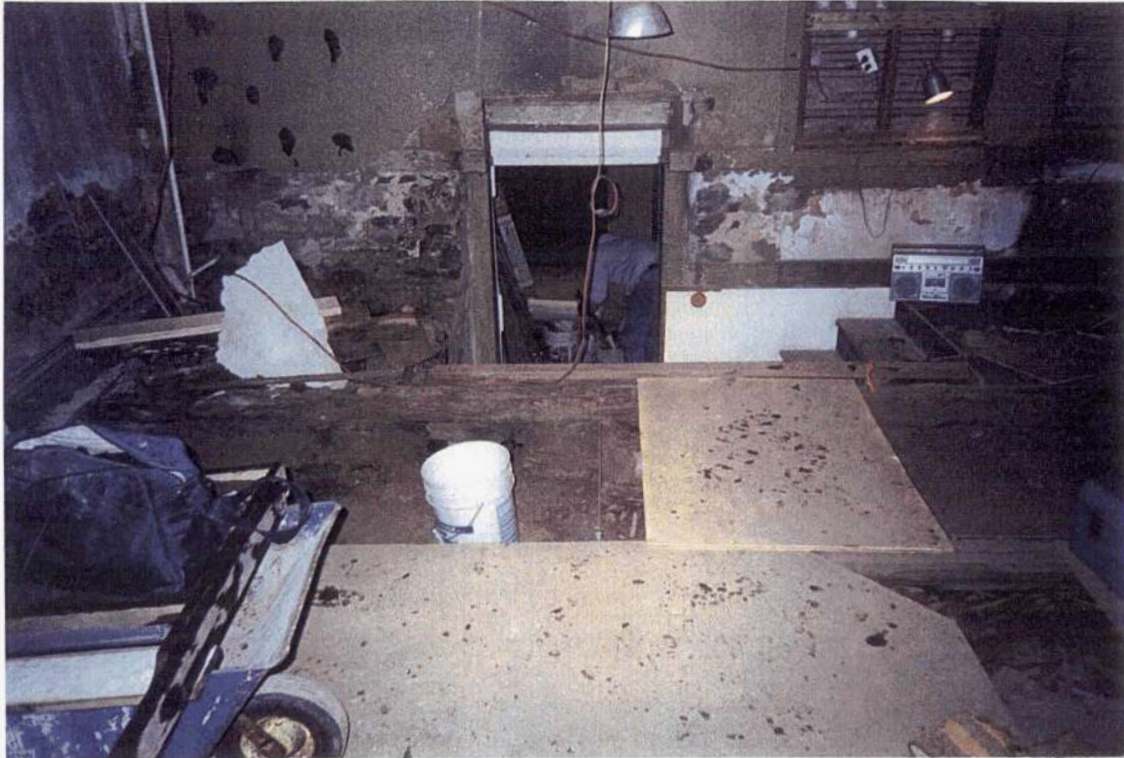
Photograph 12. Inside Phase 3, beginning of Unit 5. Basement door to Phase 2 in rear of photo. View West.
